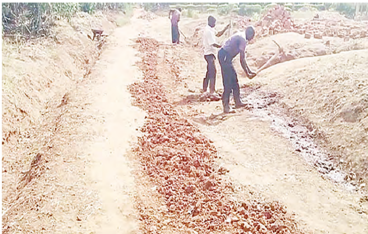
A section of rural Kaliua residents mobilised to rehabilitate a road destroyed by heavy rains. File photo.
