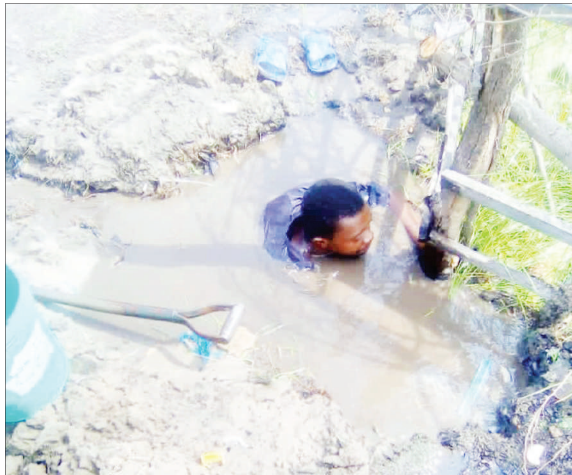
Dar es Salaam Water and Sanitation Authority technician Juma Tingisha has a rough and tough time - deep in muddy water - fighting to fix a defective pipe at Tegeta in Kinondoni District yesterday. Photo: Guardian Correspondent
