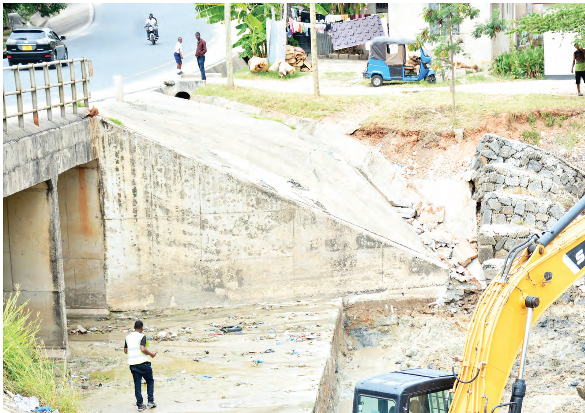
Work to clear debris blocking the flow of rainwater in progress at Mbezi River near the Makongo Bridge in Dar es Salaam yesterday. Photo: Correspondent Miraji Msala
