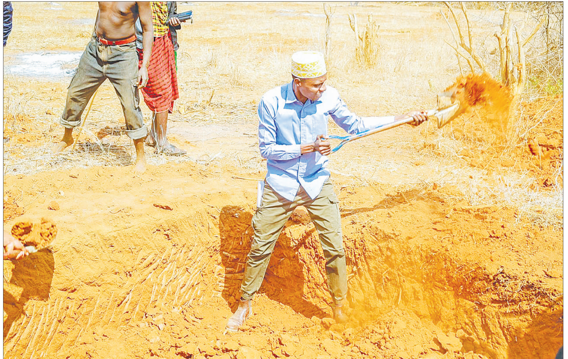
Kiteto district commissioner Remidius Mwema lends a hand in the initial stages of the construction of a building at new secondary school in Makame Ward to which the government has allocated 584m/-. Photo: Correspondent Gift Thadey
