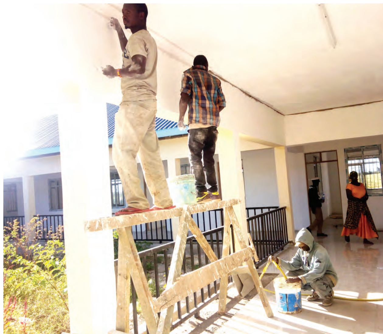
Painting in progress yesterday on buildings at Ngorongoro District Hospital, where construction is yet to be completed. Photo: Correspondent Woide Shizza
