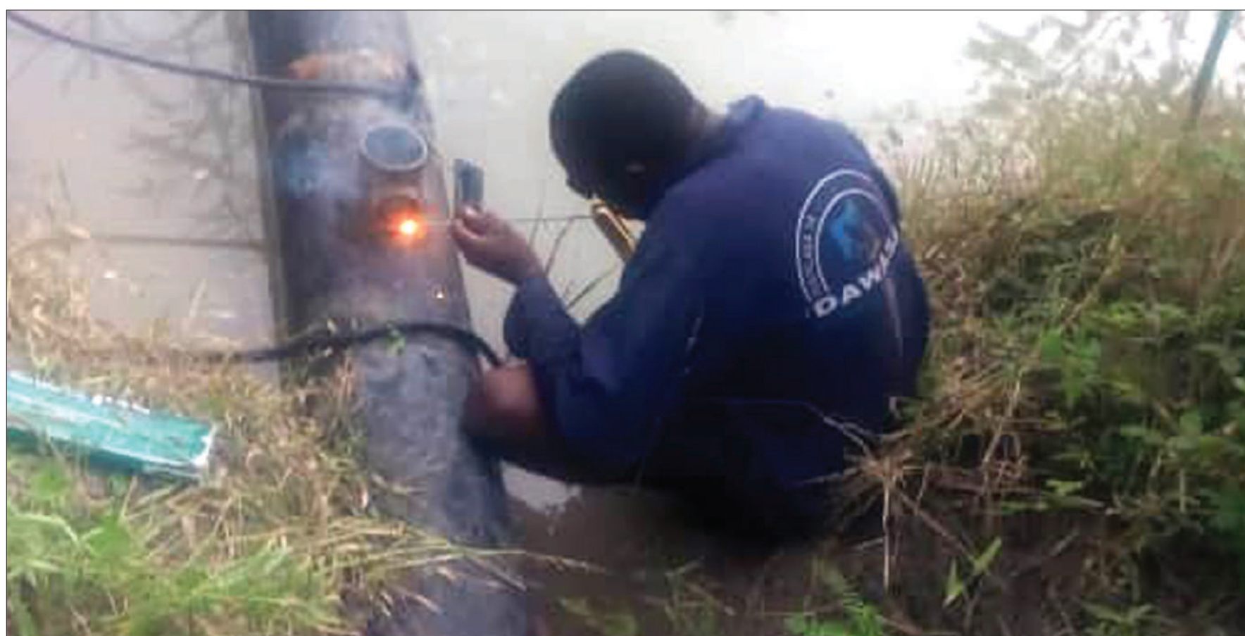
A Dar es Salaam Water and Sanitation Authority (Dawasa) technician repairs a pipe distributing water from the Changanyikeni reservoir to Kibululu and Goba suburbs in Kinondoni District, as found at the weekend. Photo courtesy of Dawasa
