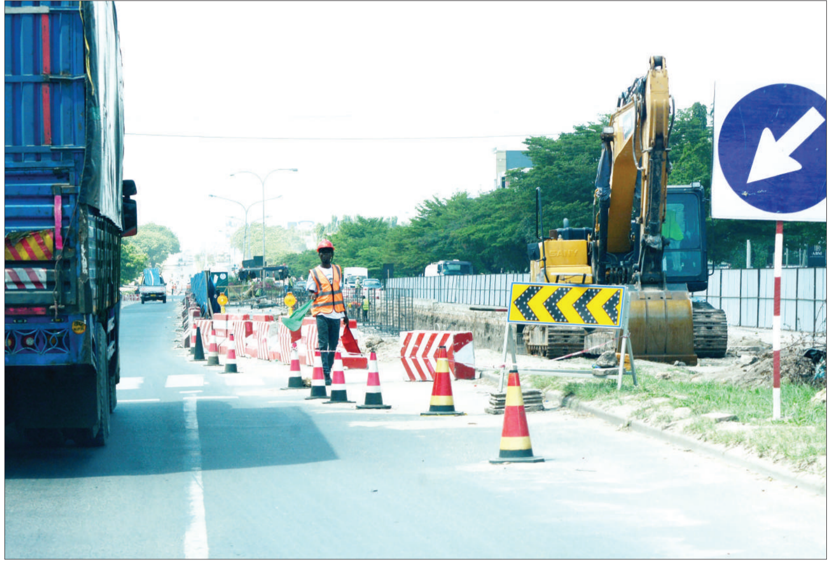
Implementation of the third phase of Dar es Salaam city's Bus Rapid Transit project has begun in earnest along the Banda la Ngozi stretch of Nyerere Road, as captured yesterday. Photo: Correspondent Jumanne Juma
