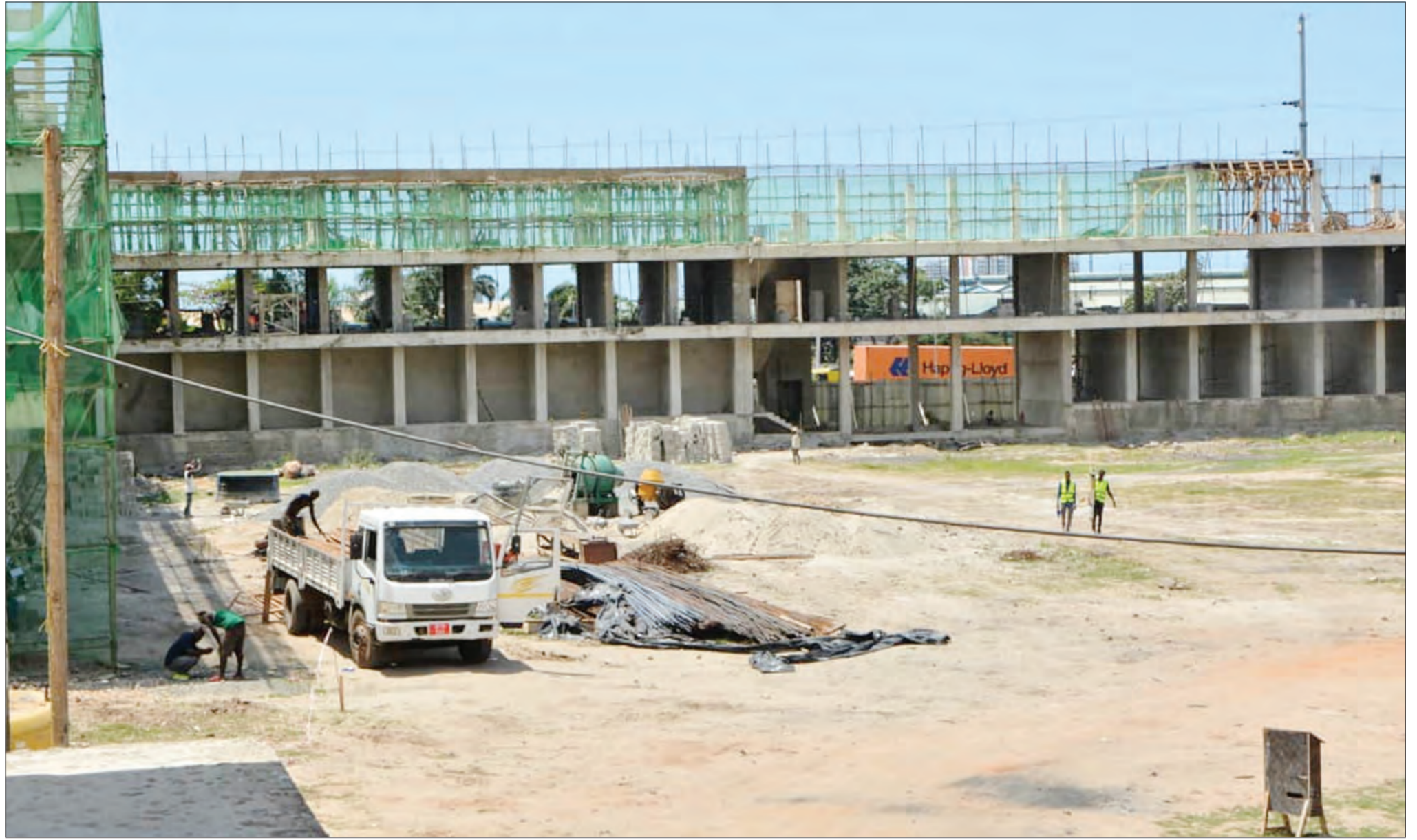
The construction of Mwenge bus stand project ongoing in Kinondoni Municipality, Dar es Salaam Region yesterday as captured by our Guardian photographer. Photo: Correspondent Mirajji Misala
