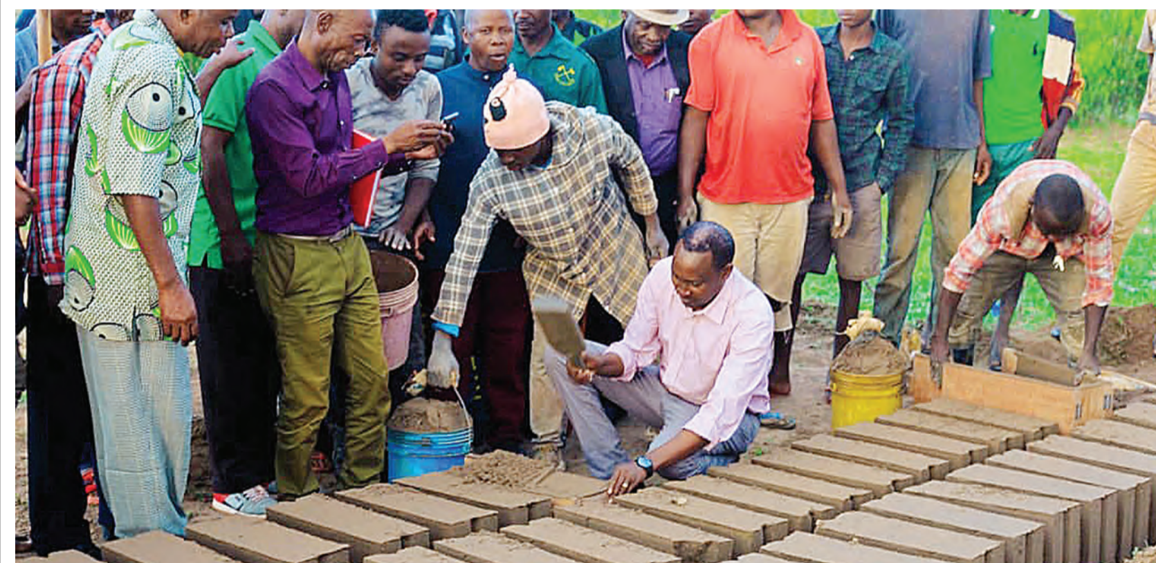
Kiteto legislator Edward ole Lekaita (squatting) joins residents of Sorongine village in the constituency's Chapakazi ward on Thursday in making bricks for the construction of a health centre. Photo: Correspondent Gift Thadey
