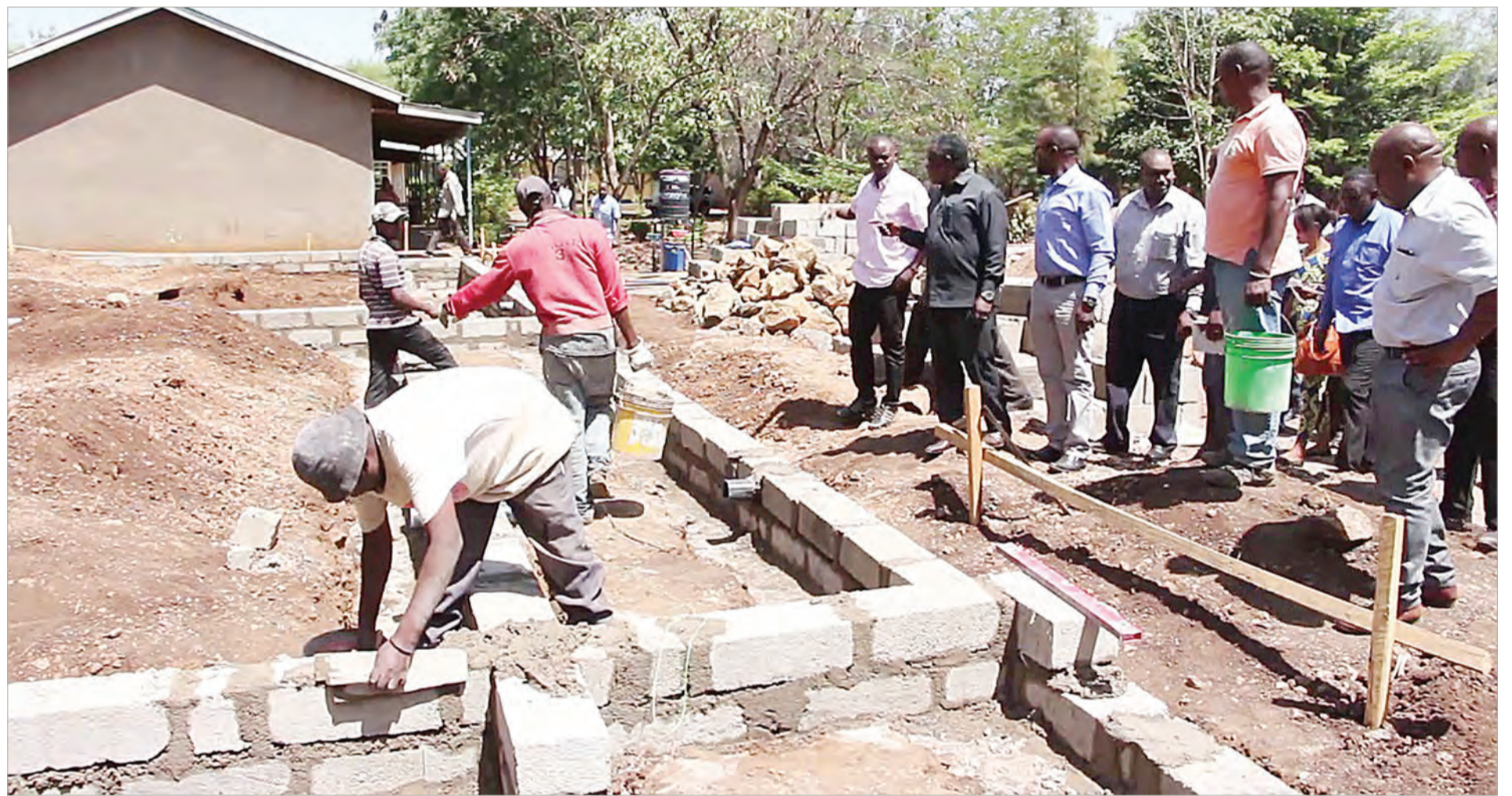
Construction of classrooms at a school meant for special needs students gets under way at Patandi in Arumeru District, Arusha Region, as found yesterday. Photo: Correspondent Getrude Mpezya
