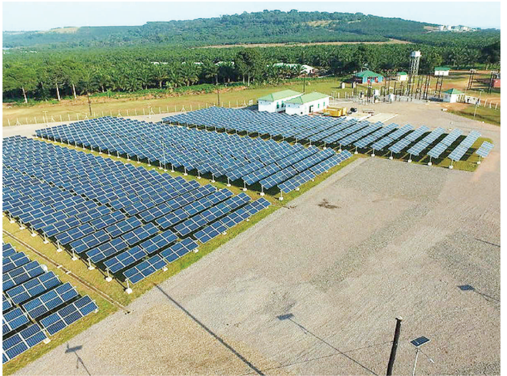
Kalangala 1.6 MW Solar-Thermal hybrid power station
