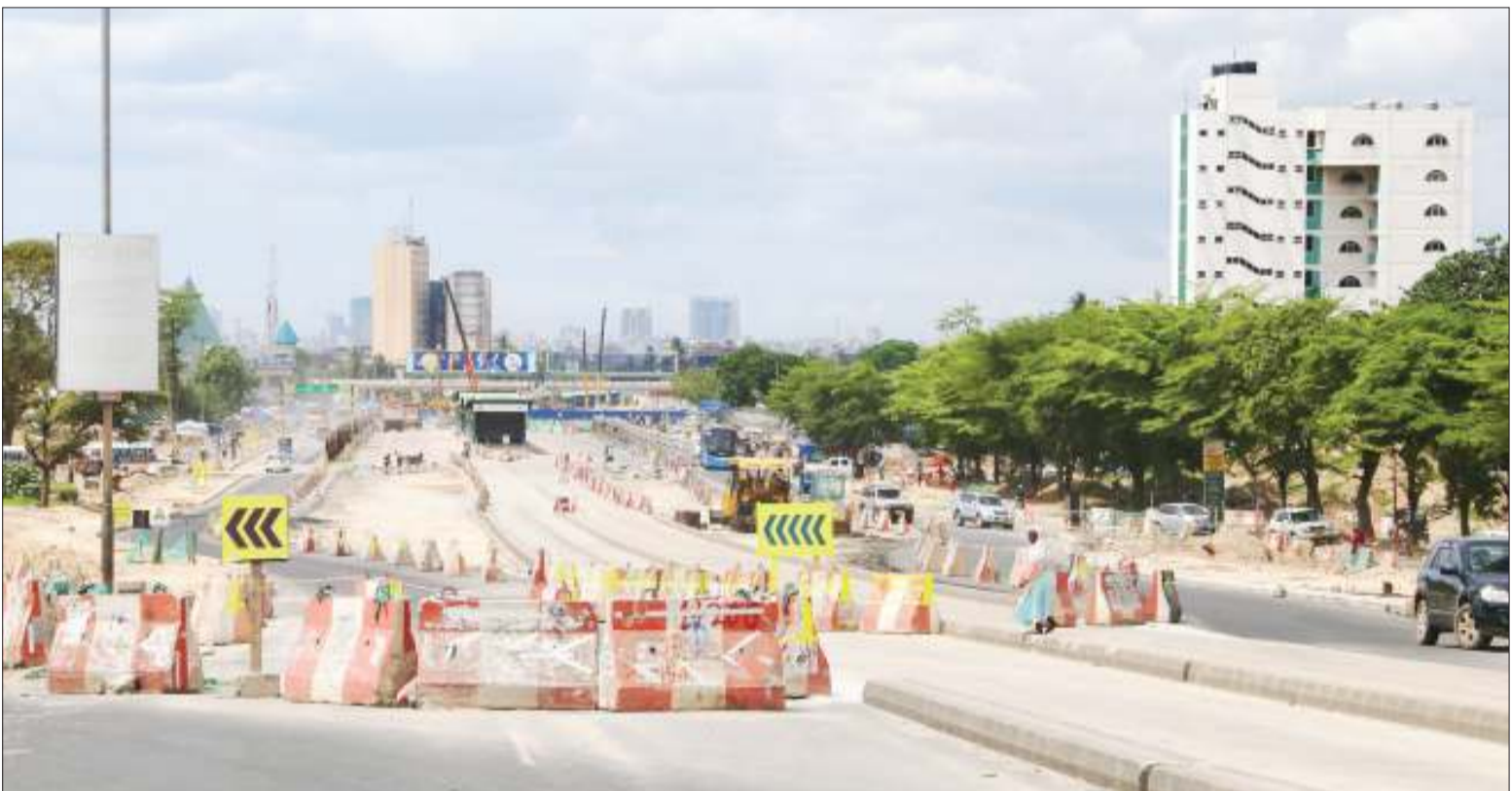
Construction of Dar es Salaam's Ubungo Interchange is making steady progress under China Civil Engineering Construction Cooperation contractors, whose ingenuity is credited with having vastly - some say magically - eased traffic jams at the Morogoro Road/Mandela Road. Chief Photographer Selemani Mpochi captured this scene yesterday.
