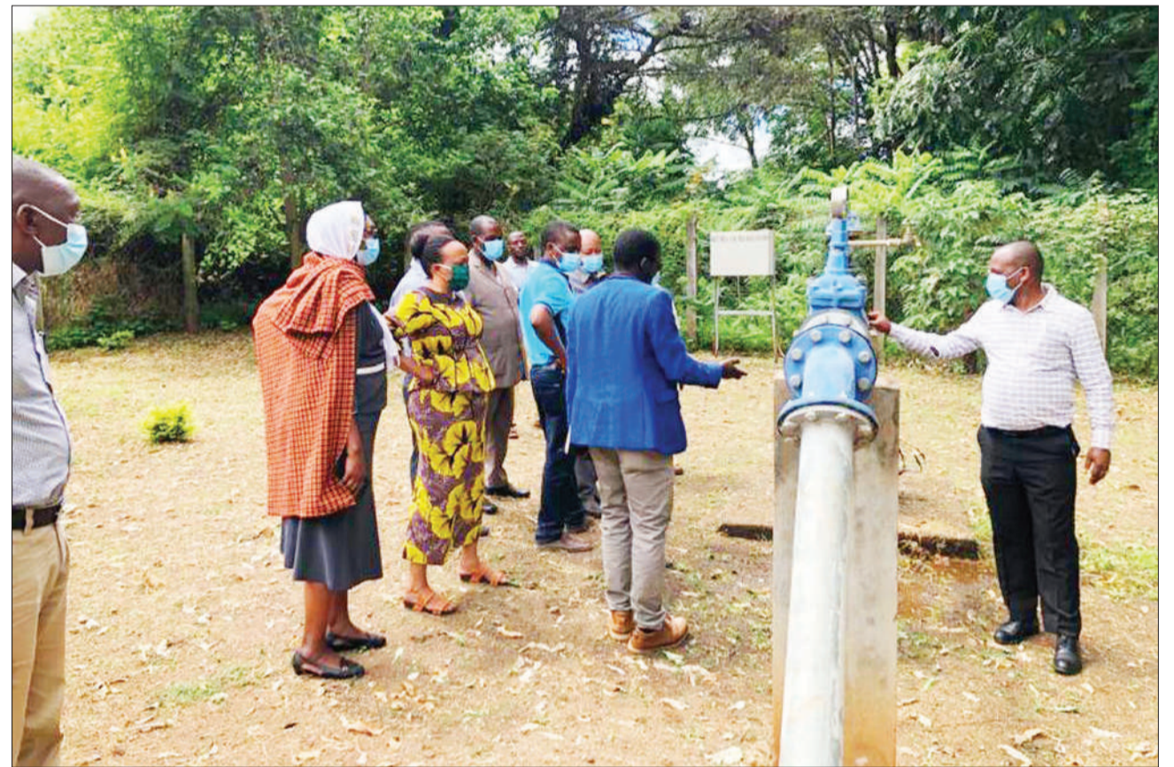
A Babati District water department employee pictured earlier this week inspecting water infrastructure, including pipes, following customers' complaints about allegedly inflated bills. Photo: Correspondent Gift Thadey
