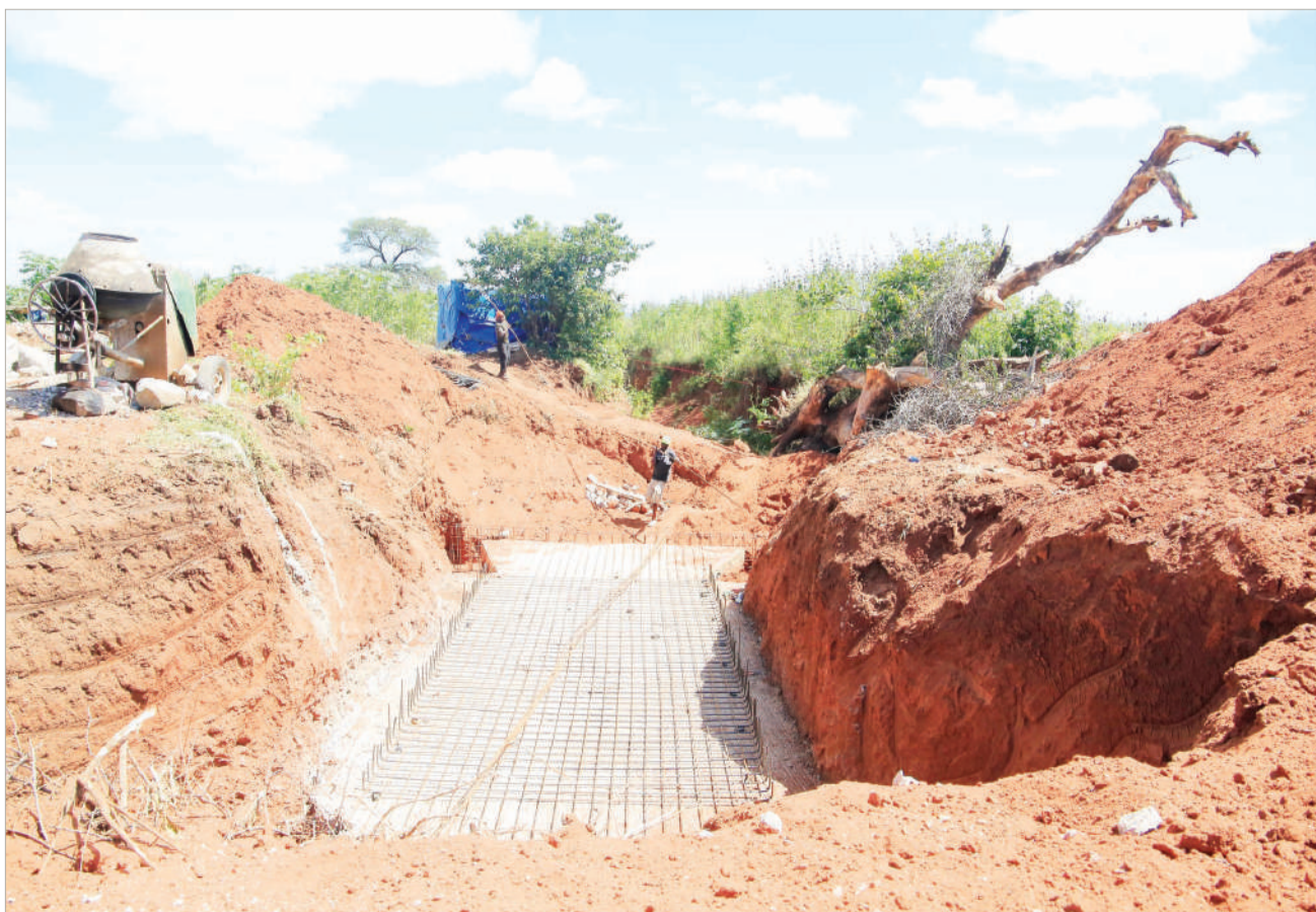
The construction of a culvert along the Bashay-Endaguday-Hydom-Yaeda Chini road in Manyara Region is well in progress, as captured yesterday. The one previously there was swept away by floodwaters recently. Photo: Guardian Correspondent
