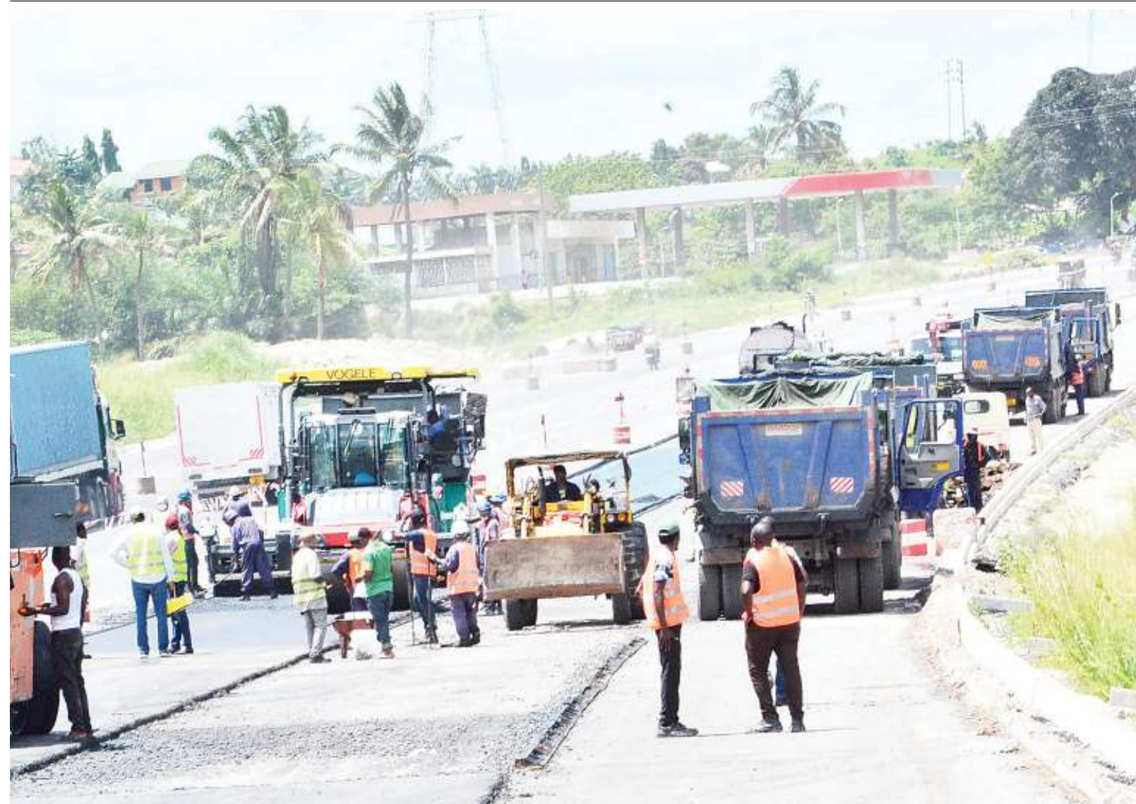
Expansion of the Morogoro Road stretch into a six-lane dual carriage way from Dar es Salaam's Kimara suburb to Kibaha well in progress, as found at a spot at Mbezi in the city yesterday, amid reports of endless traffic jams on the road due to the work. Photo: Correspondent Miraji Msala
