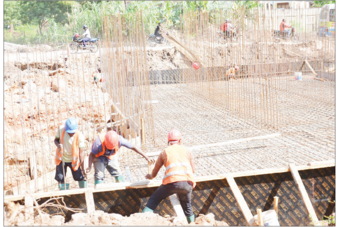
Construction of Kitunda Bridge in progress yesterday as part of the implementation of the Dar es Salaam Rapid Transit Agency (DART) road project. Photo: Nasra Hussein TUDARCO
