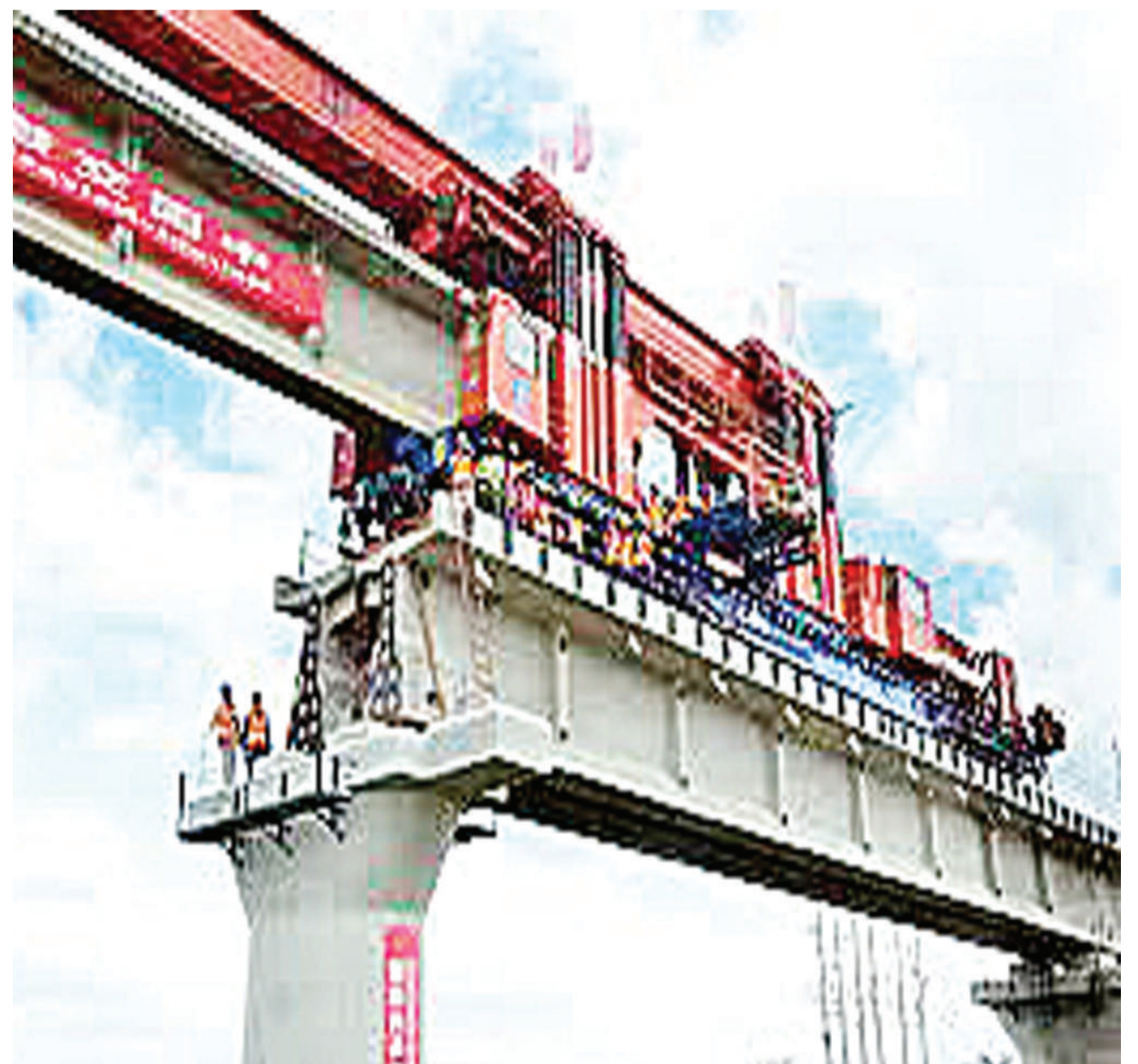
Part of SGR project currently under construction by Turkish contractor, Yapi Merkezi.
