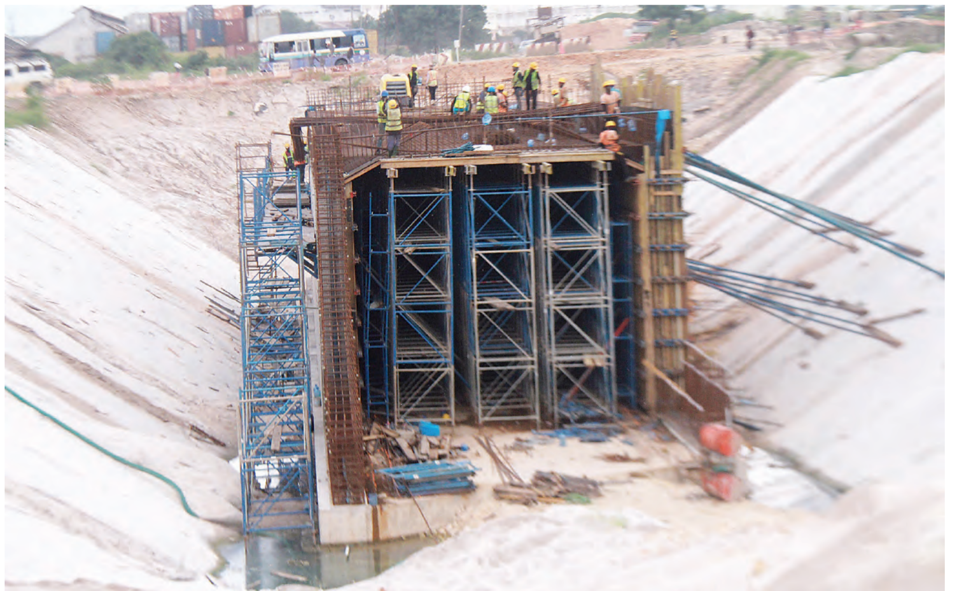
Construction of a bridge meant to keep a railway line securely separate from a road under way at Chang'ombe in Dar es Salaam yesterday. Photo: Correspondent Jumanne
