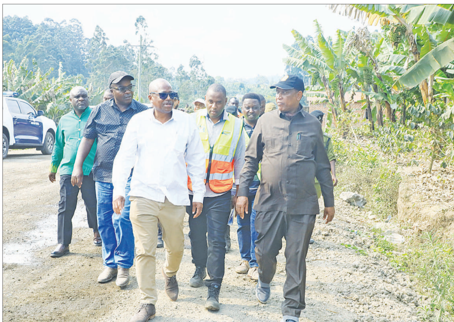
Constitution and Legal Affairs minister Prof Palamagamba Kabudi (R) makes assessment tour of progress in the construction of 8.9bn/- Ndulilo-Itete road in Rungwe District on Wednesday. In white shirt and sunglasses is Rungwe district commissioner Jaffar Hanu. Photo: Correspondent Nebart Msokwa
