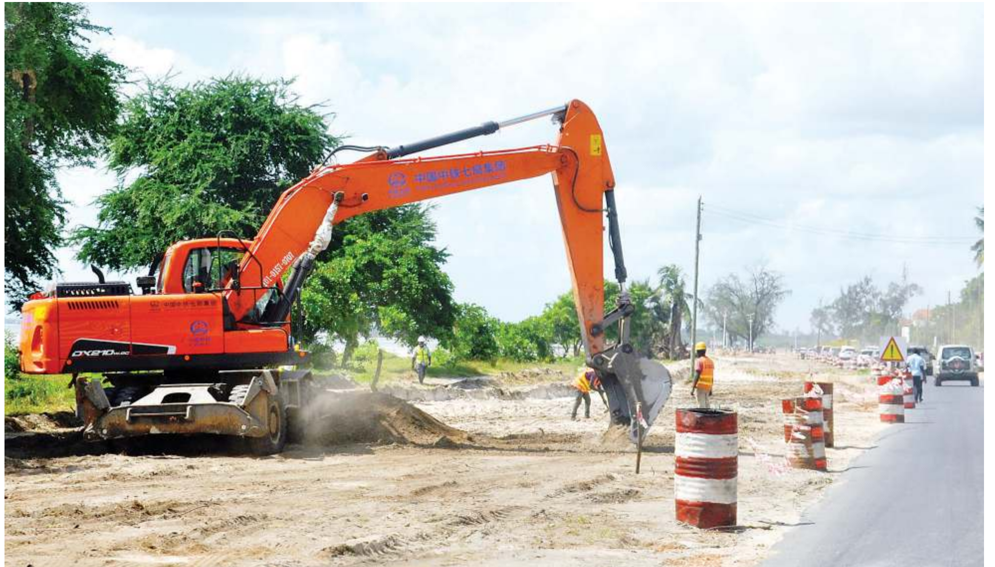
Preparatory work continues along the Aga Khan section of Dar es Salaam's Barack Obama Road yesterday to facilitate the construction of a modern bridge to link Upanga East area and Coco Beach in Oysterbay area through the Indian Ocean waters. The contractors are China Railway Major Bridges Engineering Group. Photo: John Badi
