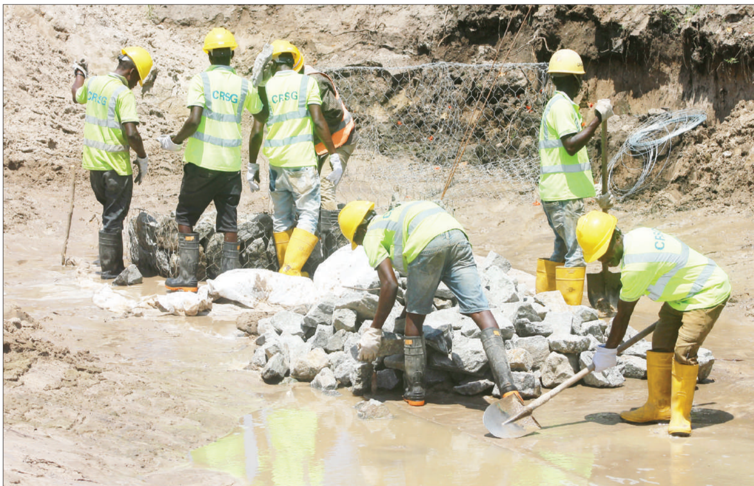
China Railway Seventh Group workers collect stones in readiness for the rehabilitation of the edges of Dar es Salaam's Chang'ombe Road, as found yesterday. Photo: Correspondent Jumanne Juma
