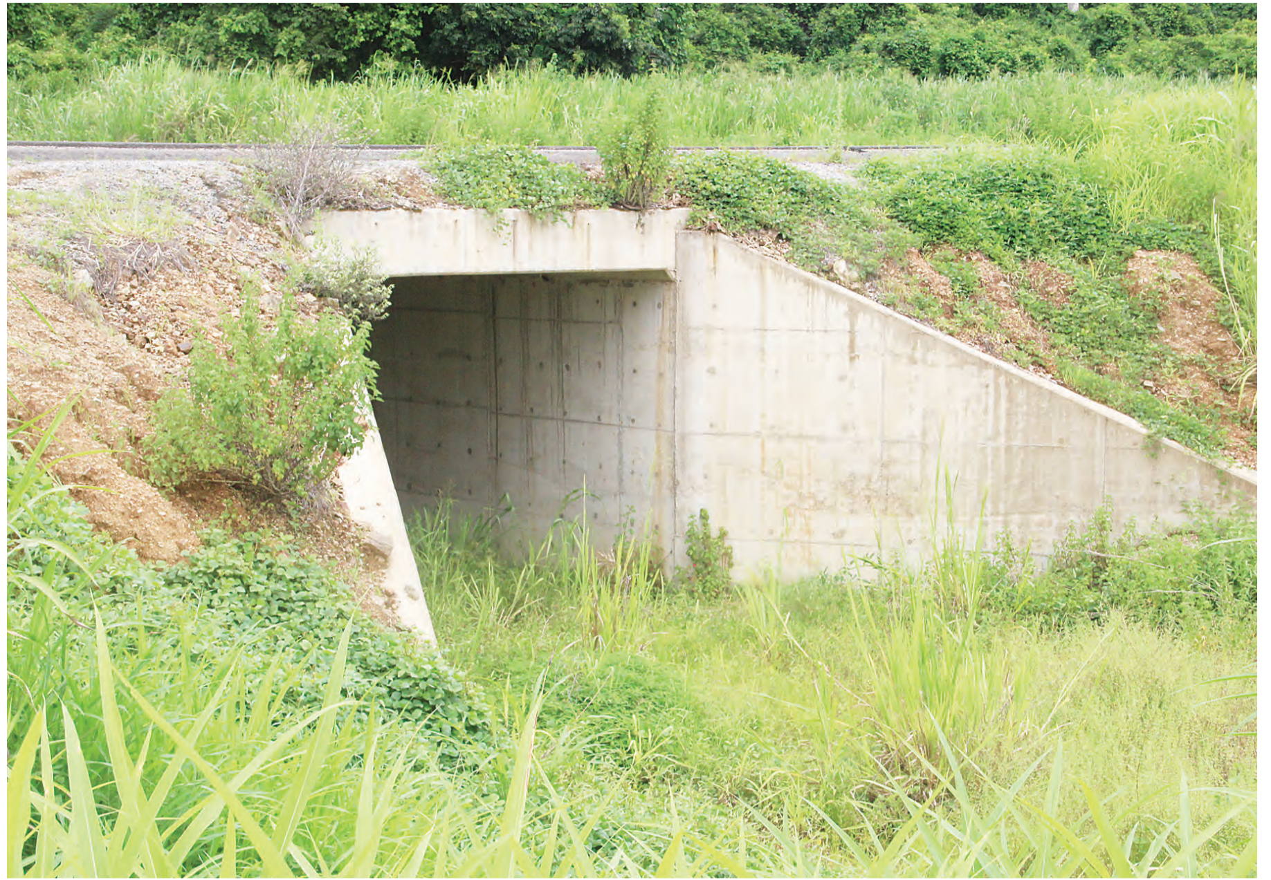
AN elephant underpass constructed along the busy Kidatu–Ifakara road in Kilombero district, Morogoro region.
