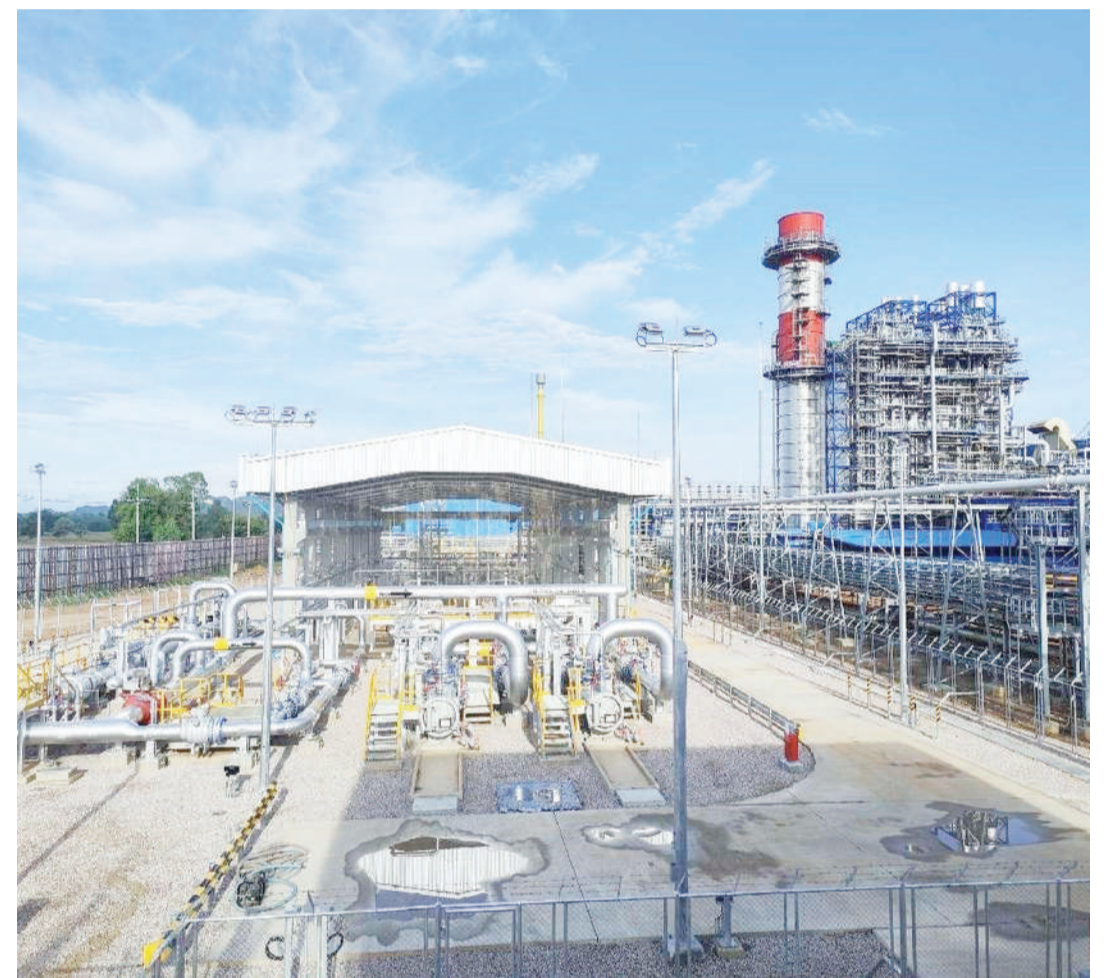
Photo shows a regulating metering station of a natural gas pipeline project built by a Chinese enterprise in Thailand. The project was put into use in September this year. (People's Daily/Sun Guangyong)
