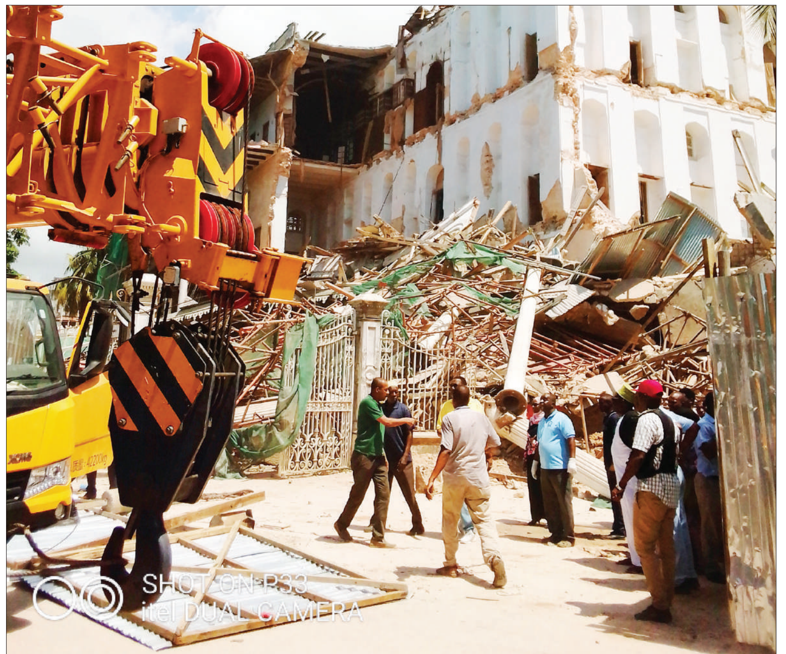
Beite-I A Jaib - the historic building which was being rehabilitated at Mjimkongwe in Zanzibar collapsed yesterday. Photo: Correspondent Martin Kabemba
