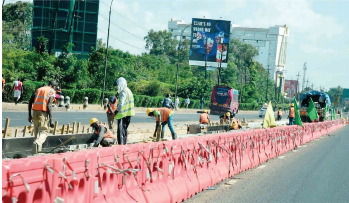
Road works for the Bus Rapid Transport (BRT) Station under construction along Thika Road Superhighway PHOTO | NM
