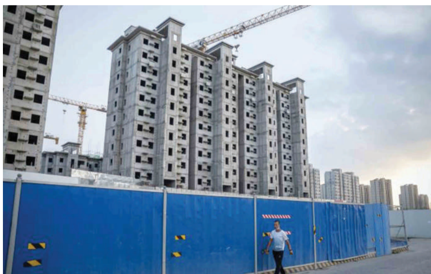
The central bank also said it would make full use of policy bank financing tools, with an emphasis on supporting infrastructure development
