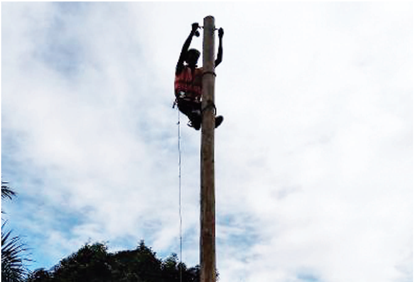
Site foreman Pius Jeremia fixes suspension cups and pig teller on an electric pole which is one of the many that will relay power to Mkeramvuti sub-location in Ilala Municipality Dar es Salaam. Photo: Beatrice Philemon.
