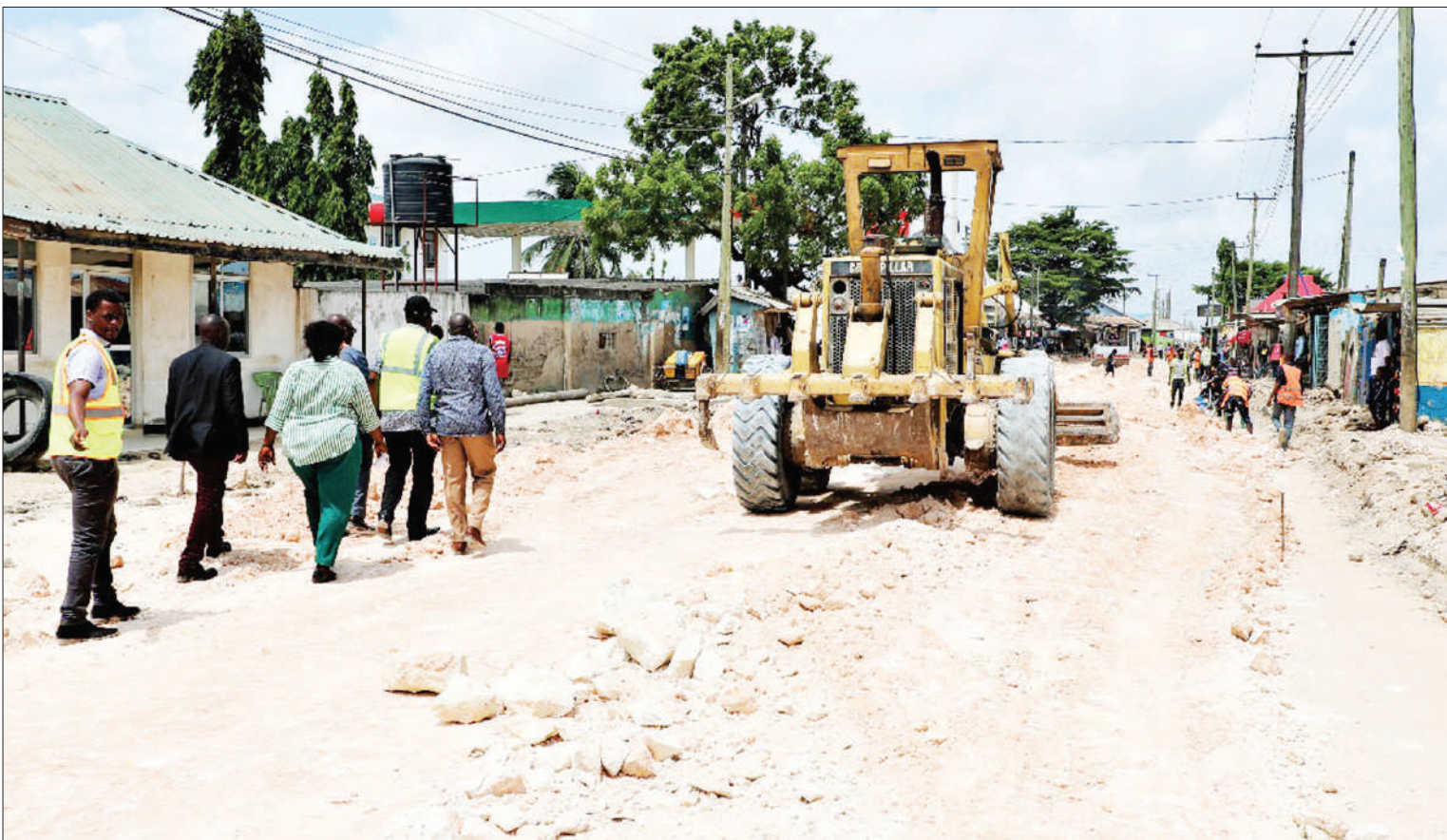
Nyanza Construction company grader levelling the ground at Vingunguti-Barakuda road in Dar es Salaam yesterday. Photo: Guardian Correspondent
