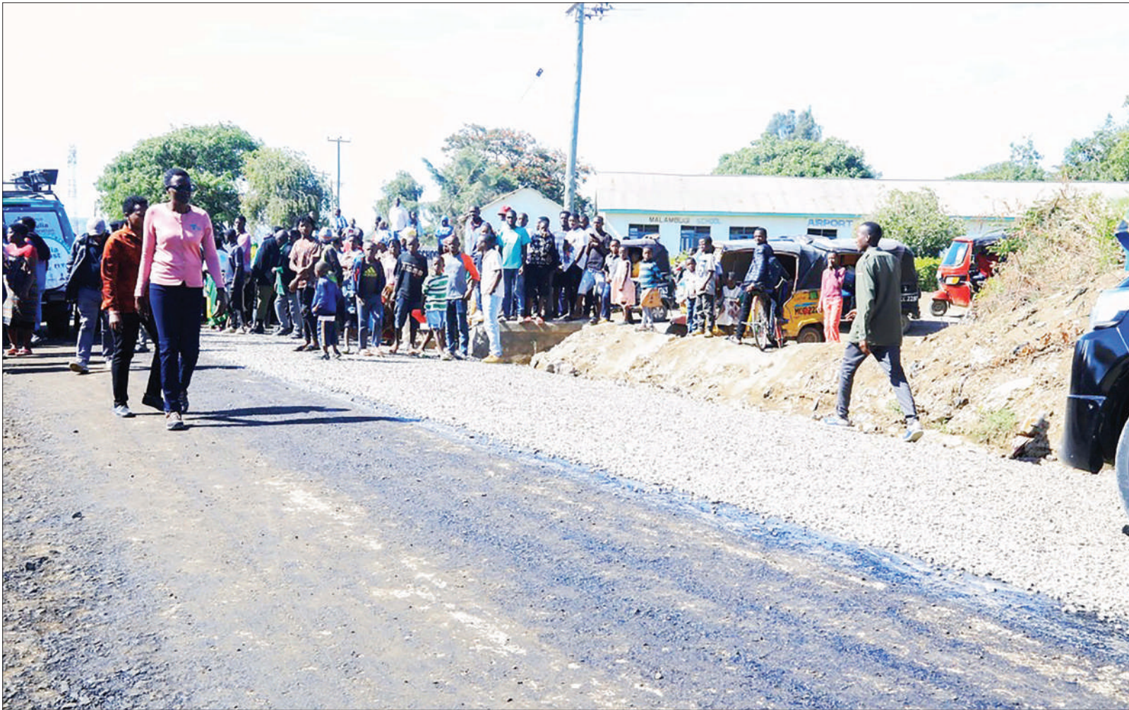
Mbeya MP who is also the Speaker of National Assembly Dr Tulia Ackson visits road construction at Iyela ward yesterday. Photo: Correspondent Grace Mwakalinga
