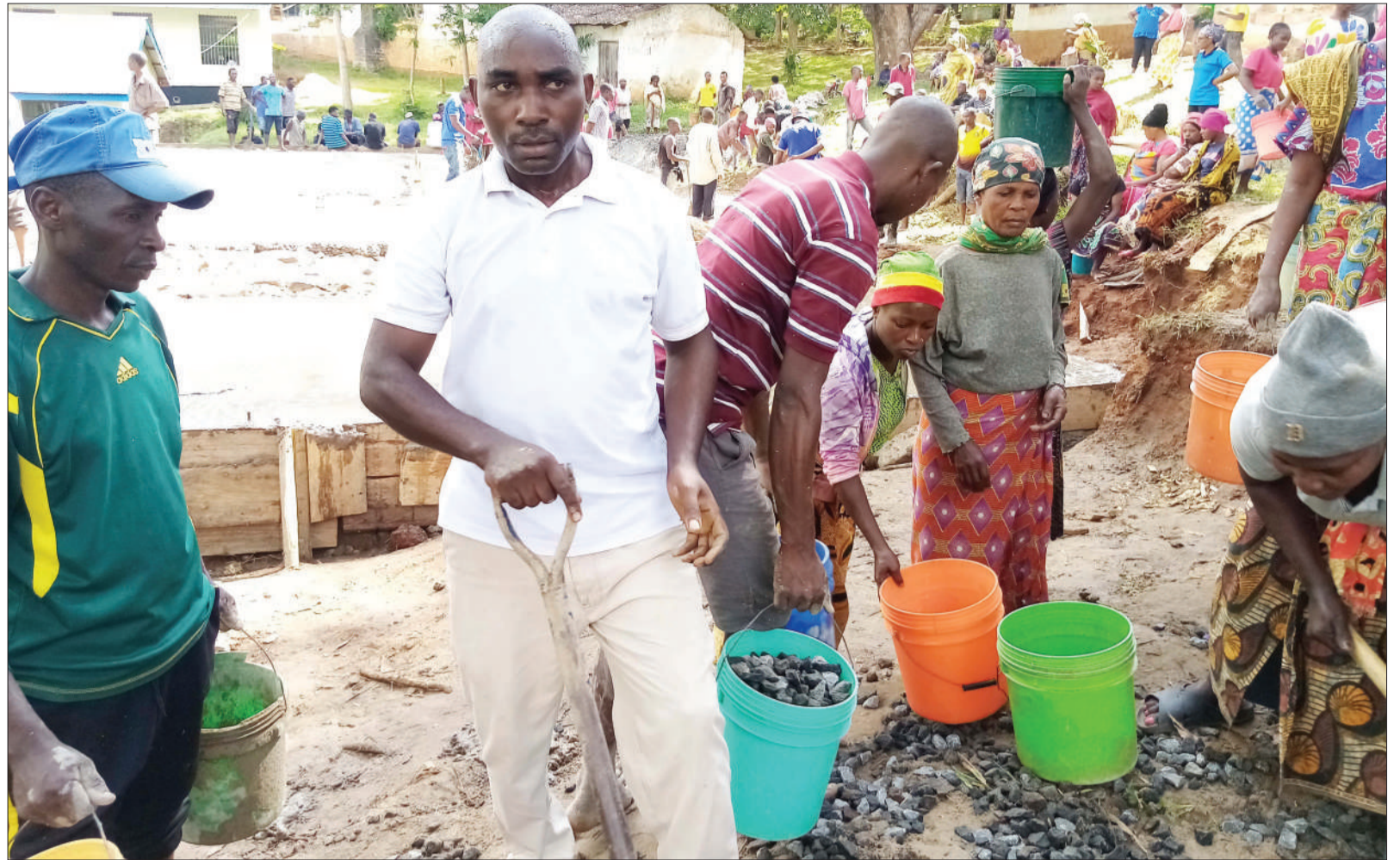
Magila residents in Muheza district, Tanga region participate in classrooms construction for Magila secondary school yesterday. Photo: Correspondent Steven William
