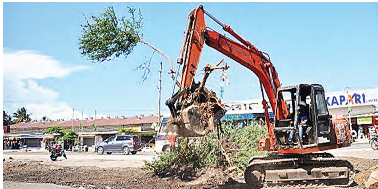
Construction goes on at Mwenge Mwisho where a main bus station for Dar es Salaam Rapid Transit buses and a four-kilometre six lane highway. File photo.
