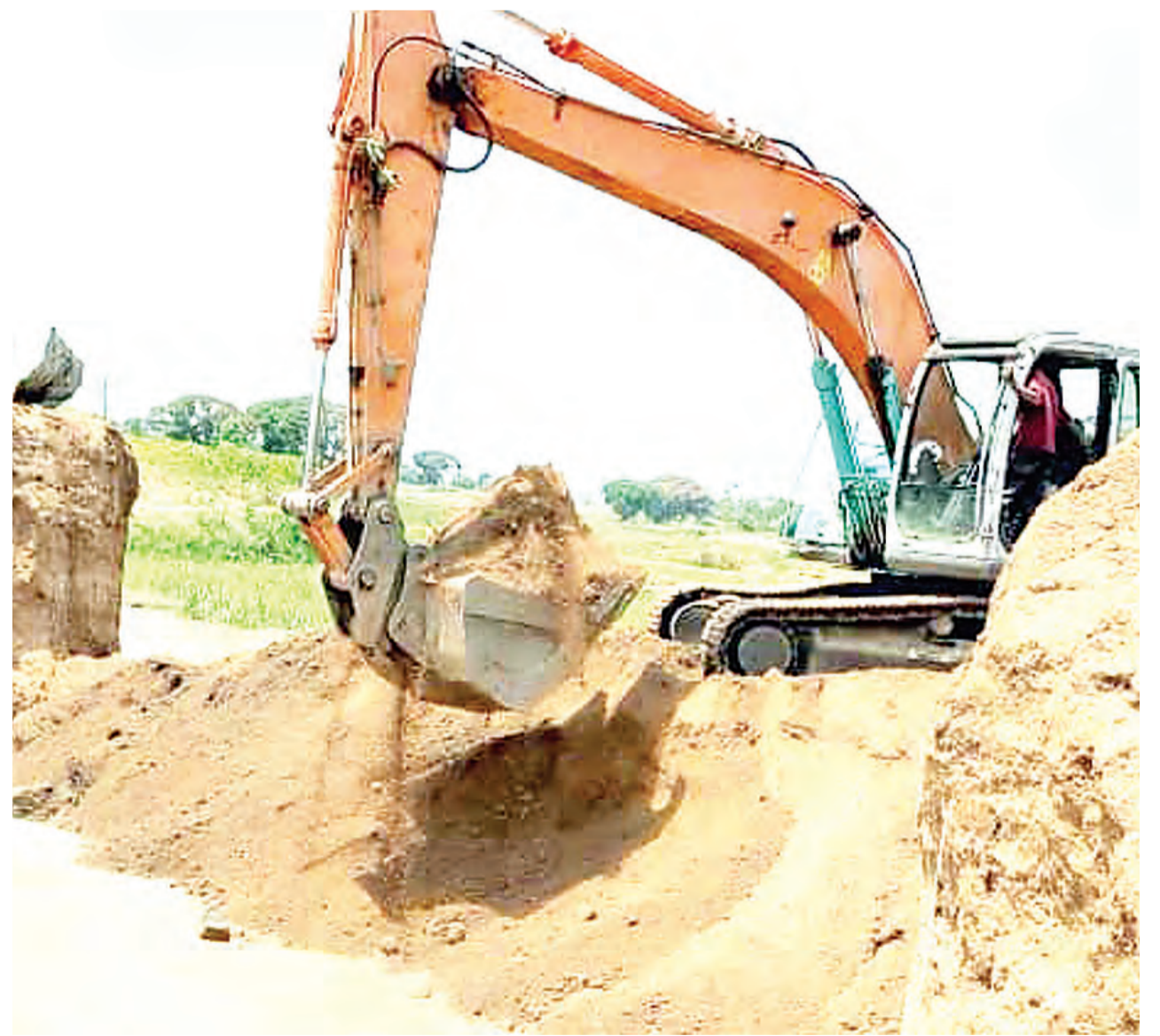
Efforts to rehabilitate Nyamwifa River bridge at Bugunda village in Musoma Rural constituency have begun in earnest, three years after days of pounding rain rendered it impassable, as found by our correspondent yesterday.
