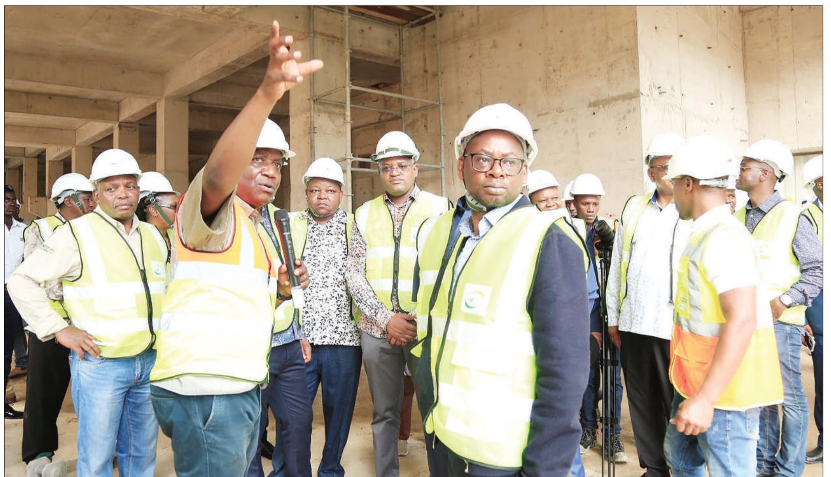
Julius Nyerere Hydro Power Project resident engineer Lutengano Mwandambo (gesturing) makes an on-site briefing to members of the project's management committee at the weekend on the implementation stage reached. Photo: Guardian Correspondent
