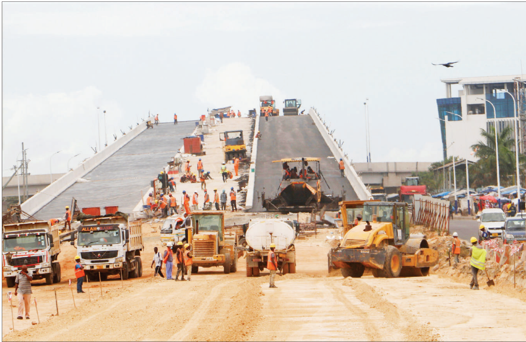
Work well in progress on the Ubungo interchange at the Morogoro Road/Mandela Road/Sam Nujoma Road intersection in Dar es Salaam yesterday. Photo: Correspondent Jumanne Juma
