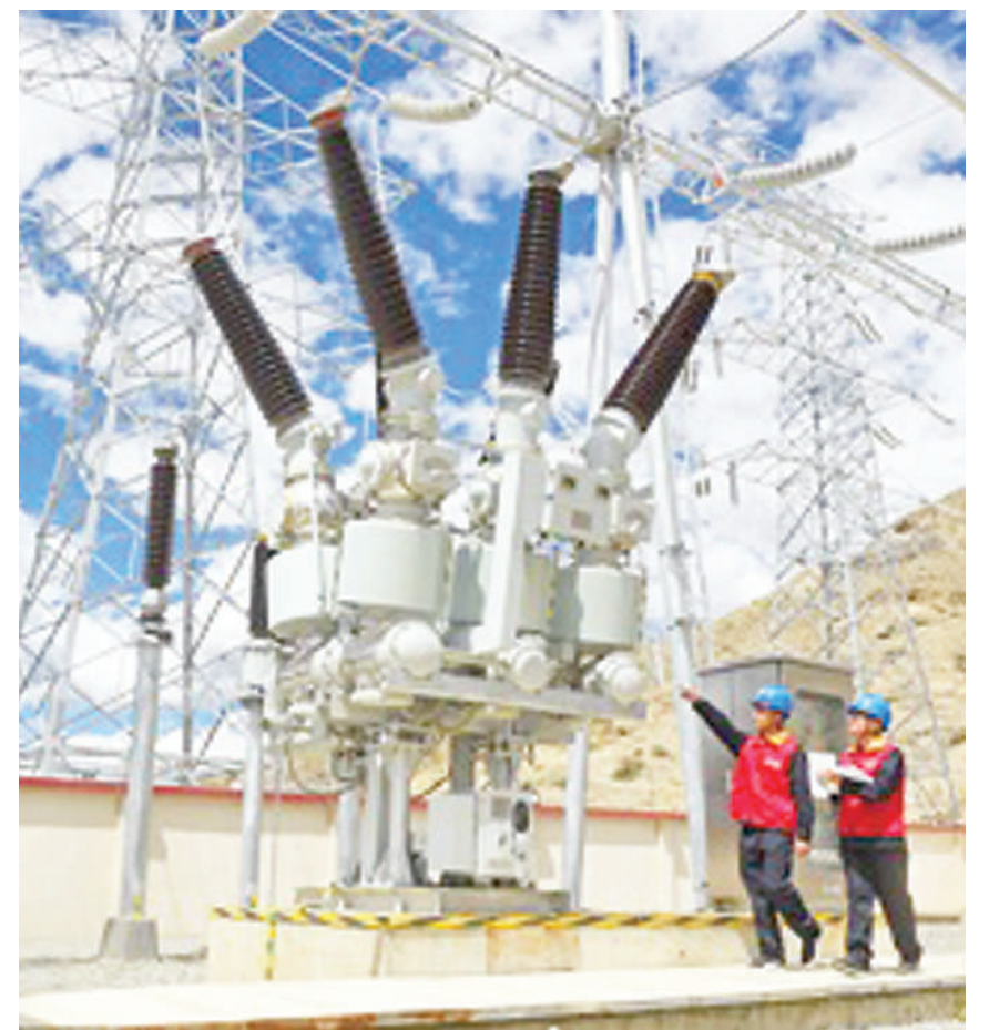
Staff workers with the State Grid Anhui Electric Power Co., Ltd. conduct inspection on power supply equipment in Zhanang county, Shannan, southwest China's Tibet autonomous region, in preparation for the peak demand for electricity in summer, June 17. File photo
