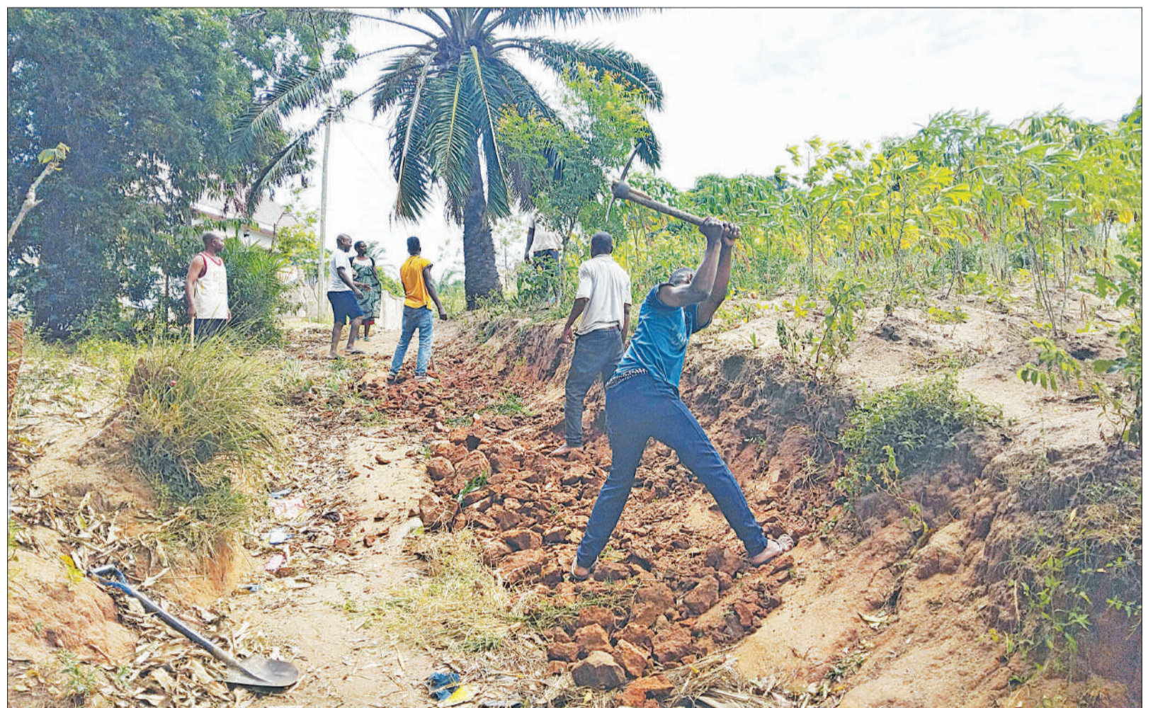
Residents of Ushuwani kwa Madawa in Dar es Salaam's Tegeta A suburb move to repair an earth road on self-help basis at the weekend. Photo: Correspondent Miraji Msala
