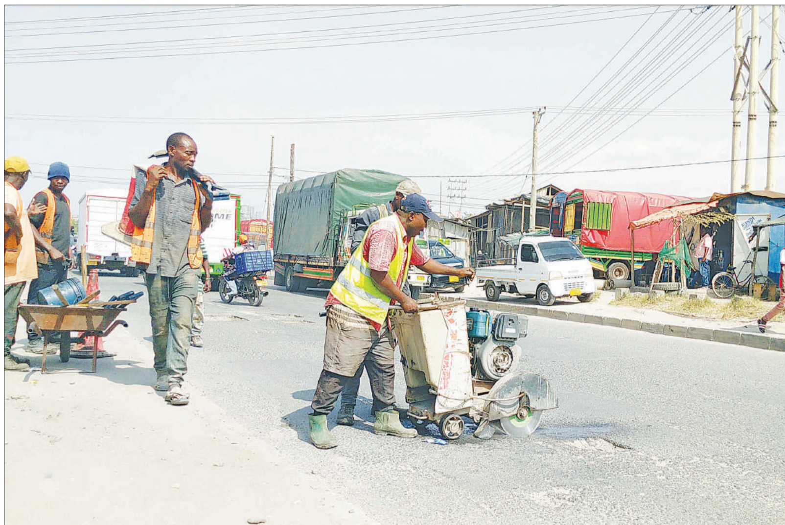
Jangwani-Mafuso section of a Dar es Salaam road undergoes repair earlier this week. Photo: Correspondent Christina Mwakangale
