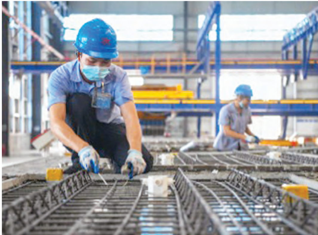
Workers are busy tying steel rods in a workshop of prefabricated building components of Hainan Weite Construction Technology Co., Ltd. based in Haikou city, capital of south China's Hainan province, Sept. 17, 2021. File photo
