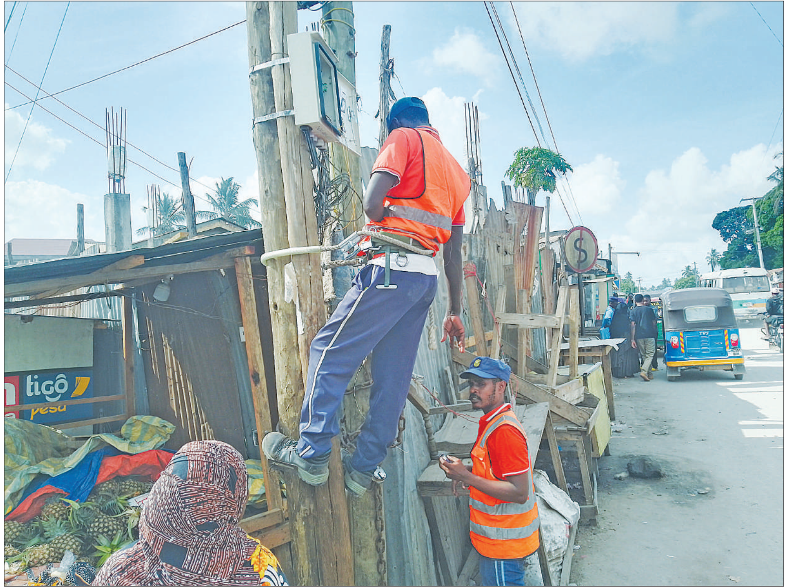
A telecommunications network technician performing maintenance on a pole at Kitunda area in Dar es Salaam yesterday. Photo: Correspondent Jumanne Juma
