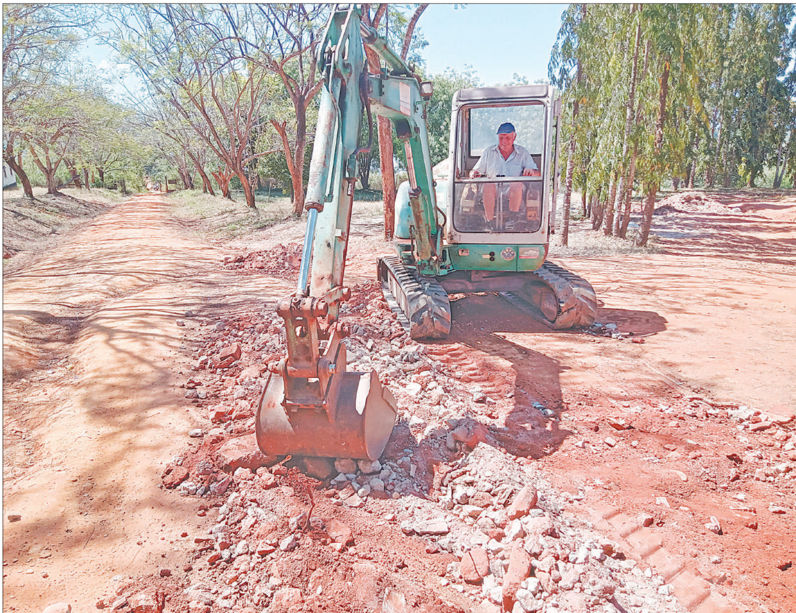
An operator for an Italian excavator levelling debris at the Passionist Fathers Missionary Church in Zeneth village in Muheza District, Tanga Region. The site was partially vacated to create space for works on the East African Crude Oil Pipeline (EACOP), where some buildings were demolished. Photo: Cheji Bakari
