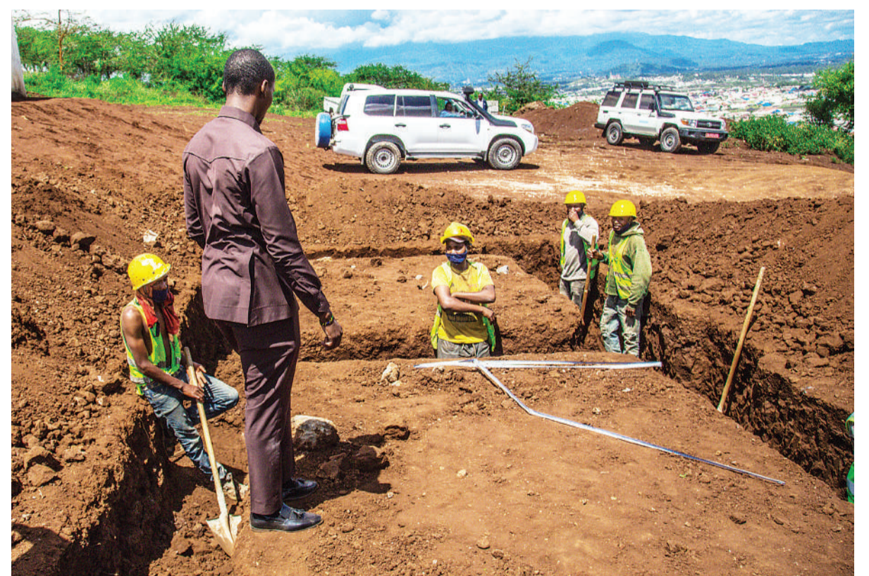
Arusha district commissioner Kenani Kihongosi (in suit) visits a water well construction site at Murieti in Olumoti ward, Arusha Region, earlier this week. Photo: Correspondent Getrude Mpezya
