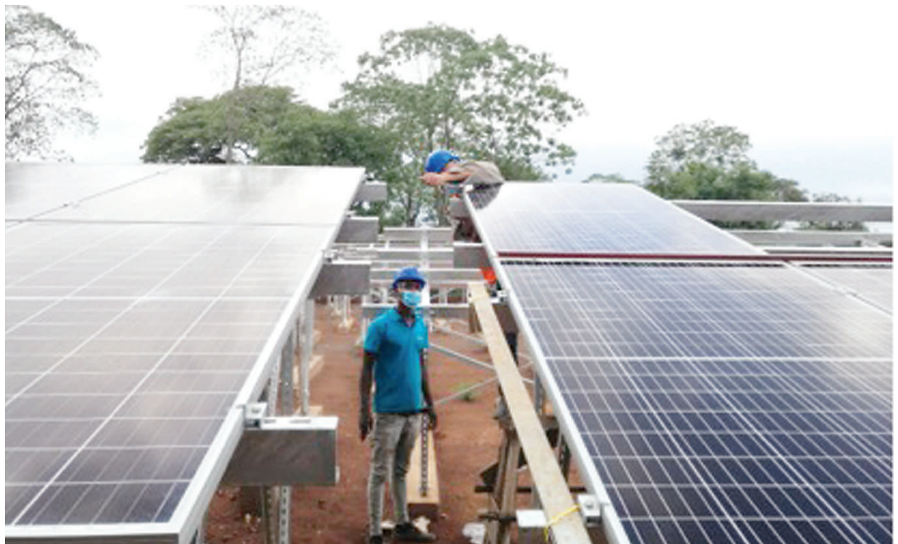
Chinese and Ethiopian workers install and adjust solar panels. (Photo/Courtesy of CET)
