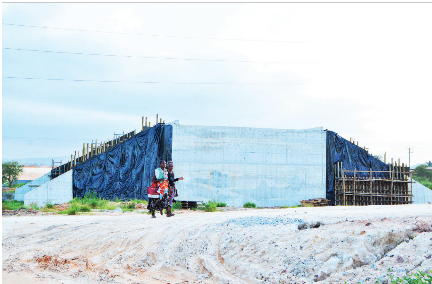
For these Dar es Salaam residents it's a stroll close to a Standard Gauge Railway bridge (to their left) under construction in the city's Gongo la Mboto Mwisho suburb, as captured yesterday. Photo: Correspondent Miraji Msala
