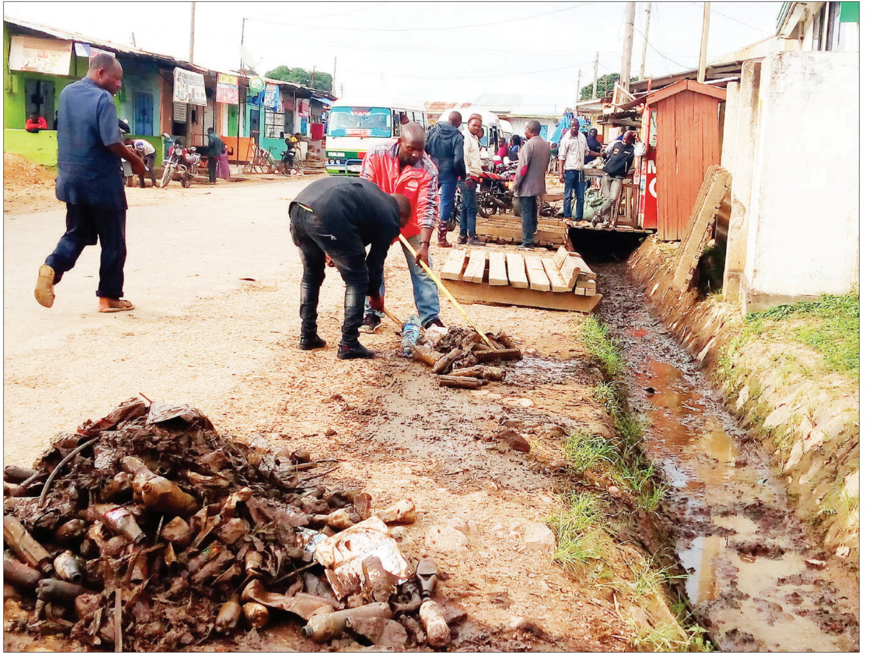
Motorbike taxi riders clear a sewage system at Mbalizi in Mbeya Region at the weekend as part of a mandatory weekly environmental cleanliness routine for the township's residents. Photo: Correspondent Nebart Msokwa
