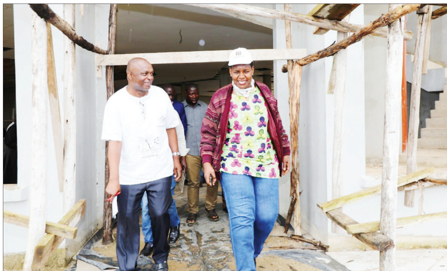
Lands, Housing and Human Settlements Development deputy minister Dr Angeline Mabula (R) and Missenyi district commissioner Col Denis Mwila on an inspection tour of a National Housing Corporation investment building under construction at Mutukula on the Tanzania side of the border with Uganda at the weekend. Photo: Correspondent Munir Shemweta
