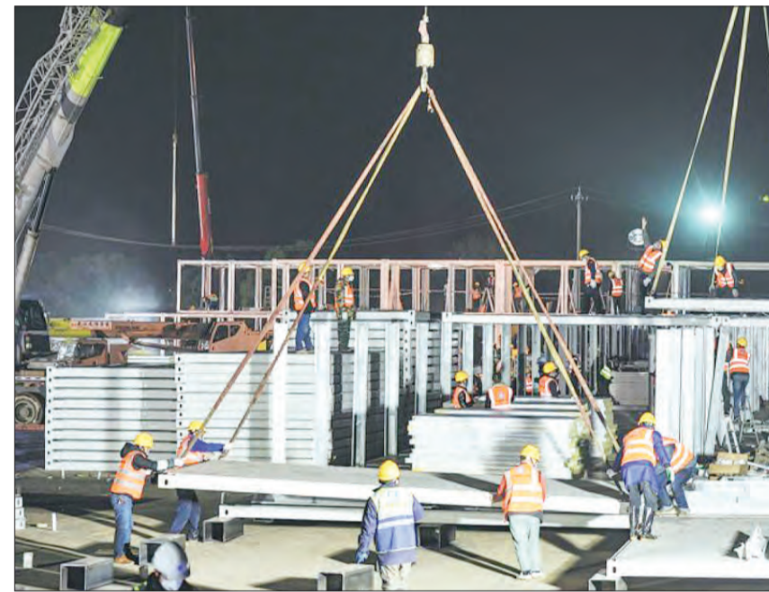
Workers bring the pieces together. Work is expected to be done by Feb 3, about seven days after it began.
