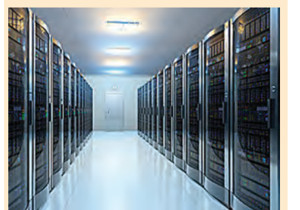
Inside Africa Data Centres facility in Midrand, South Africa.
