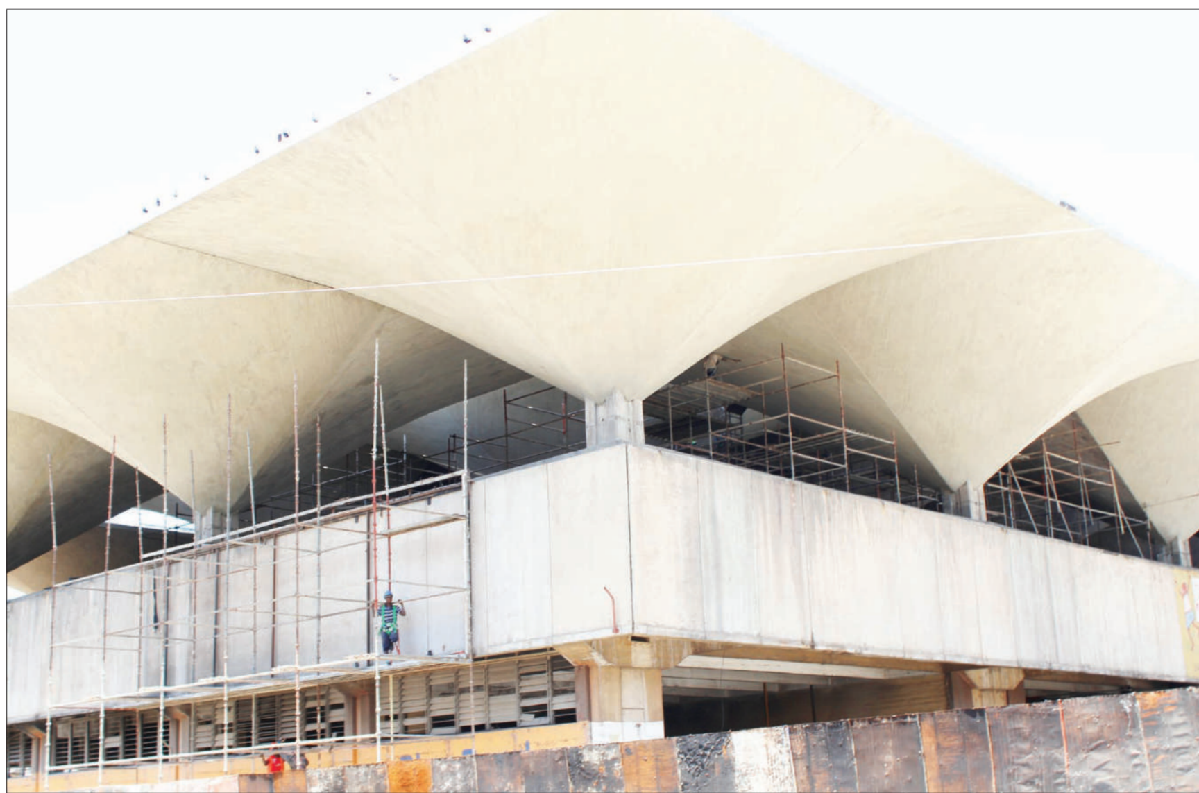
This is Dar es Salaam city's main mixed-goods market, Kariakoo, which is undergoing rehabilitation after being gutted by fire in July last year. Correspondent Jumanne Juma captured the scene yesterday.
