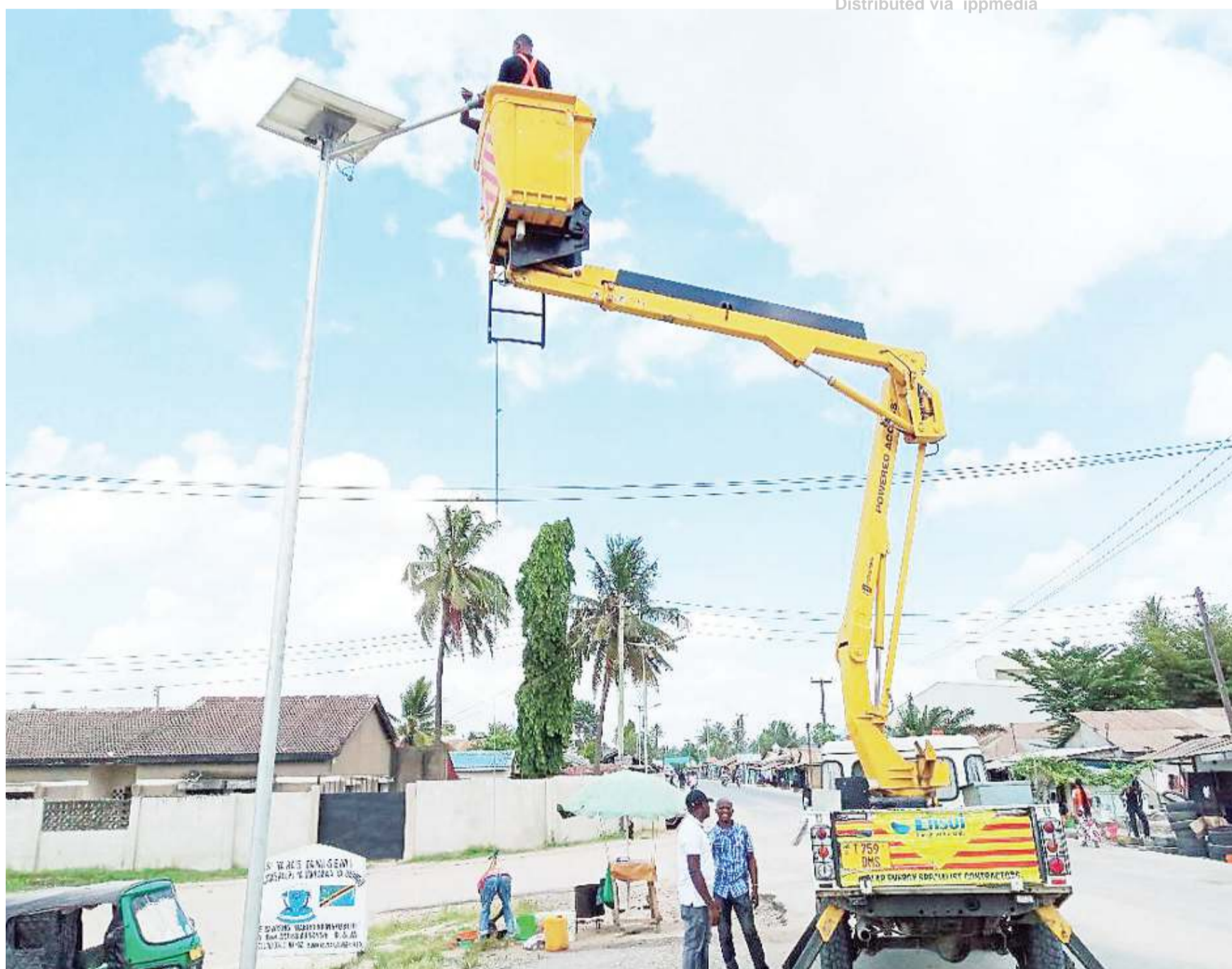
Ensol workers installing solar energy light along Tabata External road in Dar es Salaam yesterday. Photo: Correspondent Joseph Mwendapole
