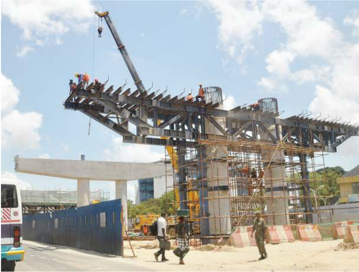
City residents walk near the ongoing construction of Ubungo Interchange at the roundabout of Morogoro Road/Mandela Expressway in Dar es Salaam yesterday. Photo: John Badi
