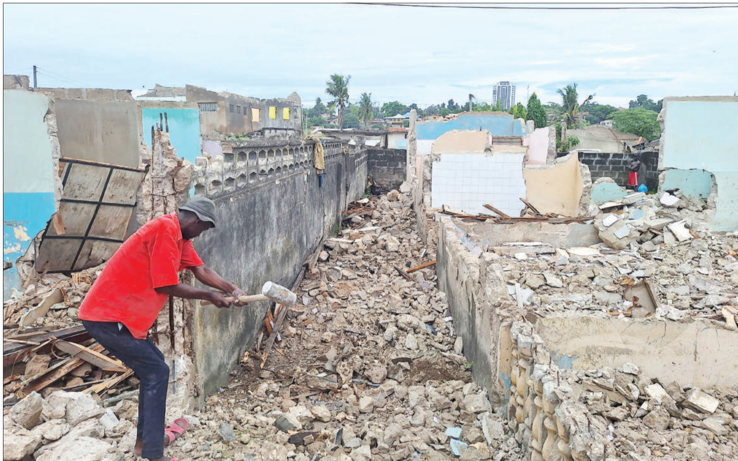
Demolition of a house standing in Dar es Salaam's flood-prone Jangwani area under way yesterday to pave the way for the implementation of the Msimbazi Valley redevelopment project. The Guardian has it on good authority that the owner of the house has already been compensated. Photo: Correspondent Joseph Mwendapole
