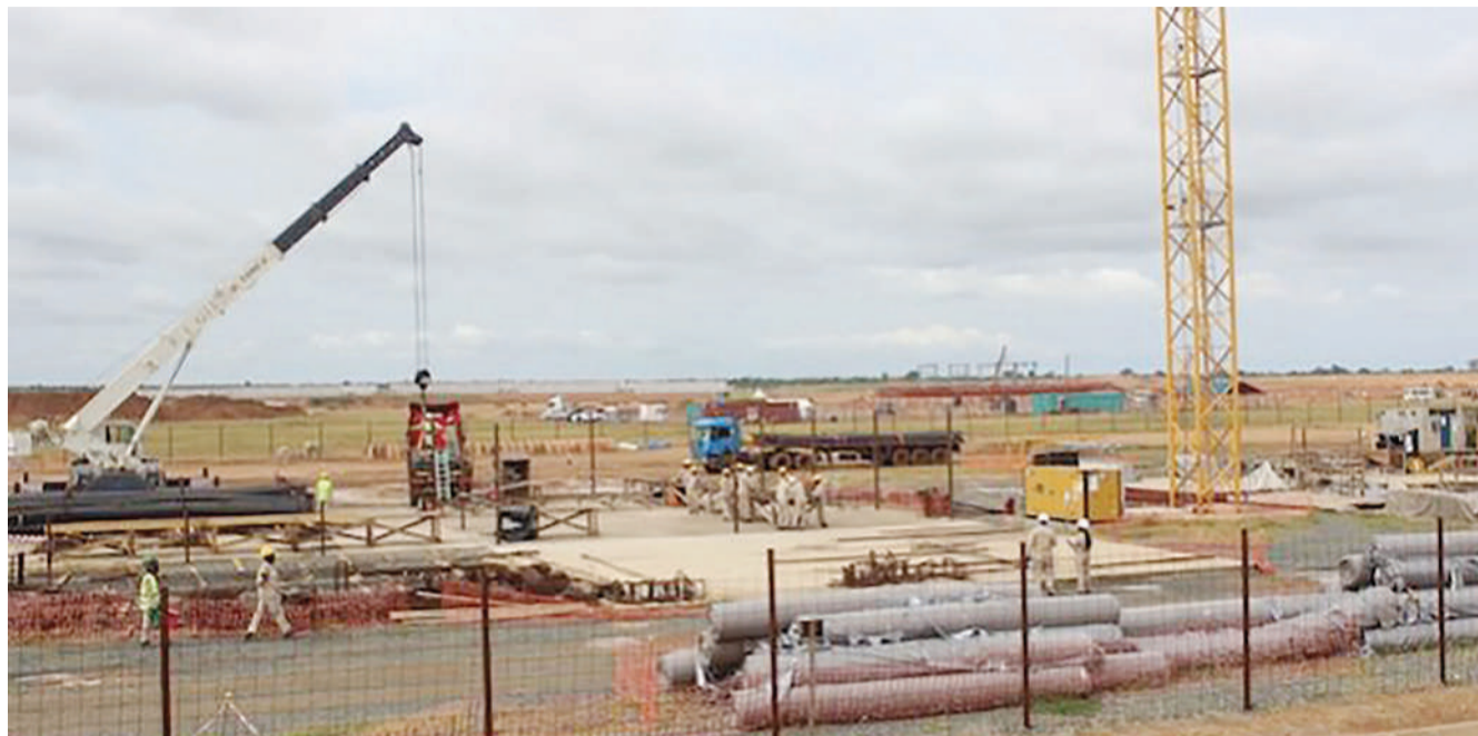
Works at the Tilenga Development Project operated by TotalEnergies. Some landowners object to what they consider forced evictions with inadequate compensation.
