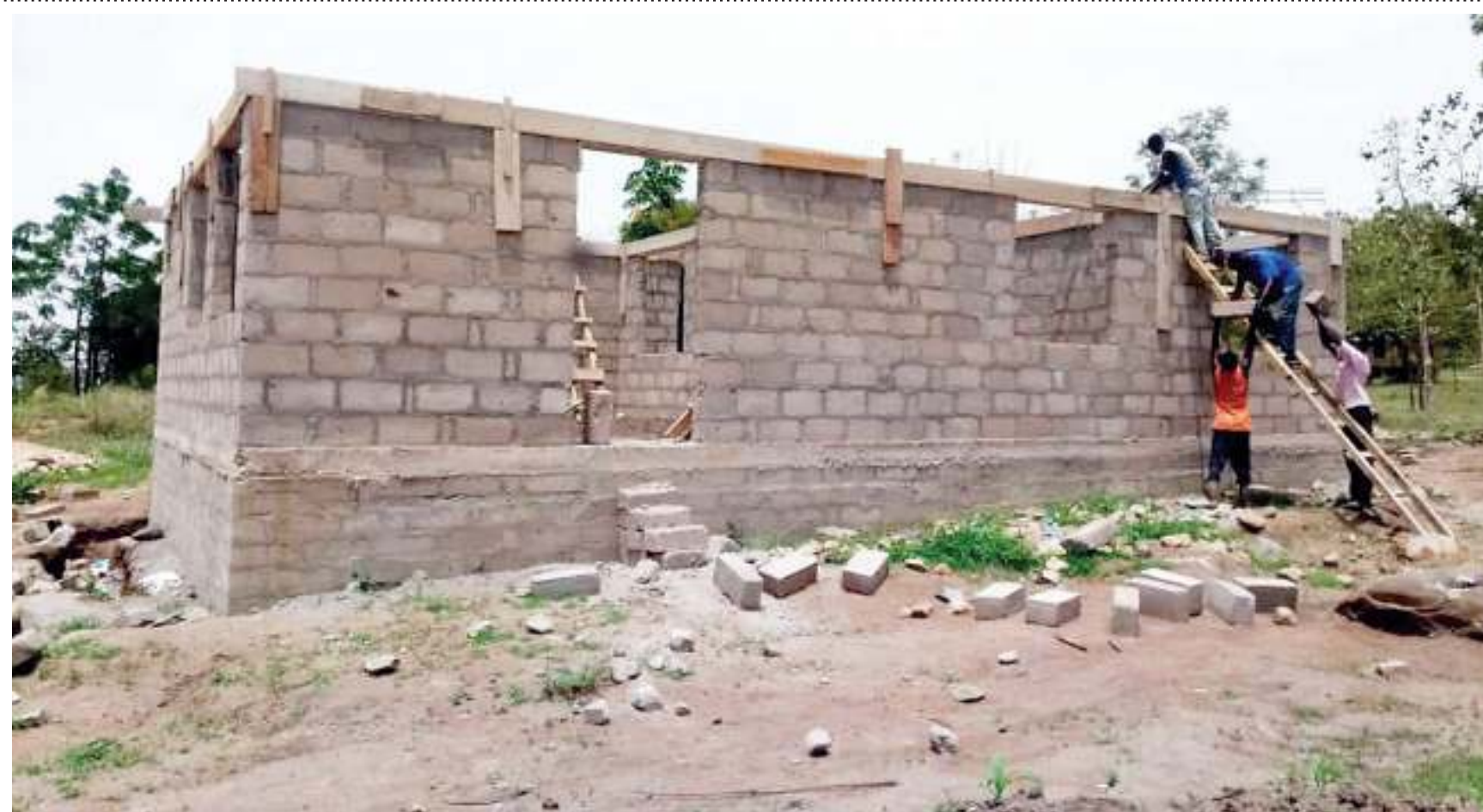
Construction of one of the houses meant as teachers' quarters in progress at the newly established Tegeruka Secondary School in Musoma Rural constituency, Mara Region, as found on Monday. The project is being implemented largely on self-help basis. Photo: Guardian Correspondent
