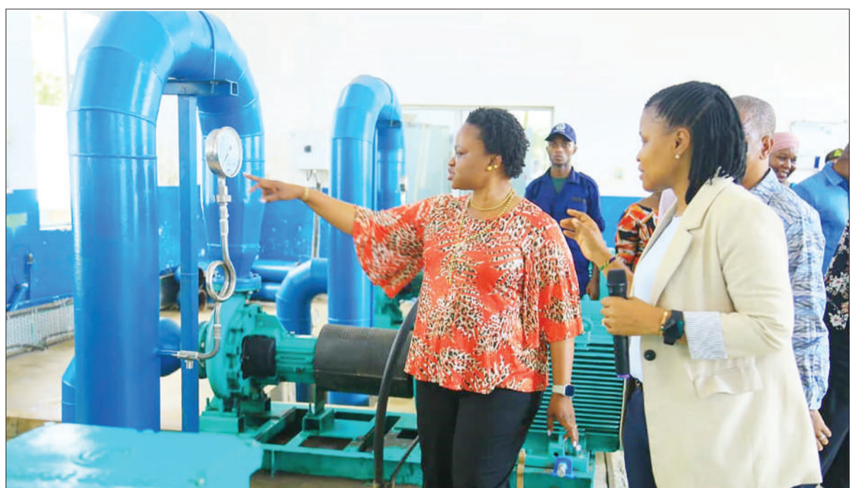
Deputy minister for Water, Engineer Maryprisca Mahundi, (L) gets a brief about the expansion of Wami water production plant from the manager of the plant, Engineer Emaculata Msilama (R) when she visited Chalinez third phase of the project yesterday. Photo Correspondent Joseph Mwendapole
