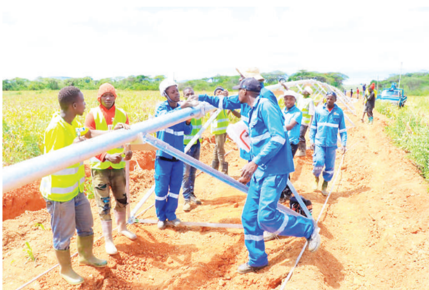
Pro Agro Global Company Ltd workers install modern irrigation infrastructure at the Kilimi Seed farm in Nzega District Tabora Region. Photo: Correspondent Valentine Oforo
