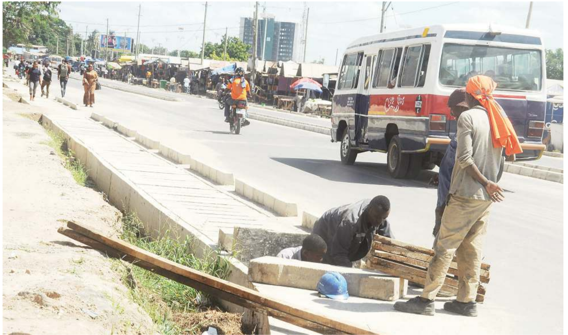
Construction of a roadside trench in progress near the Simu 2000 commuter bus stand at Ubungu in Dar es Salaam, as found yesterday. Photo: John Badi
