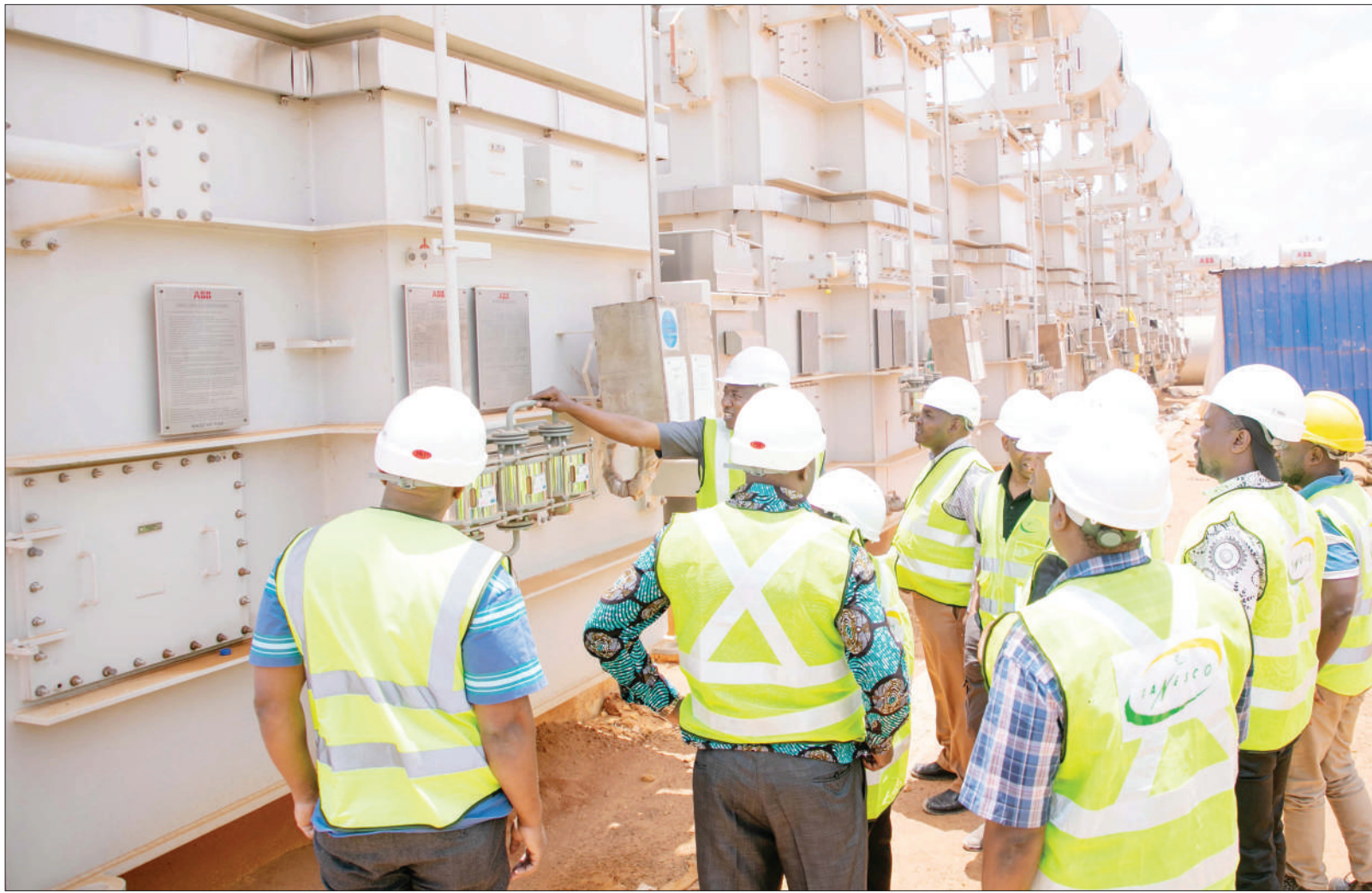
Members of the Parliamentary Energy and Minerals Standing Committee are briefed on transformers lined up for installation at the Julius Nyerere Hydro Power project site, which they toured in Coast Region at the weekend. Photo: Guardian Correspondent
