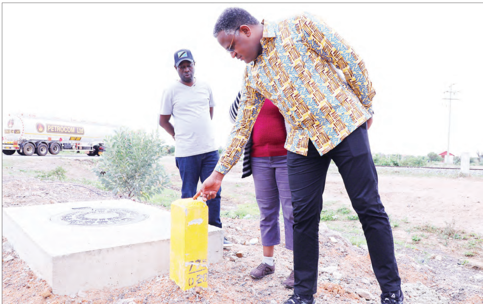
Dr Jim Yonazi (R), Information, Communications and Information Technology ministry permanent secretary, pictured yesterday inspecting national fibre-optic infrastructure for Manyoni in Singida Region to Kambikatoto in Mbeya Region. Photo: Guardian Correspondent
