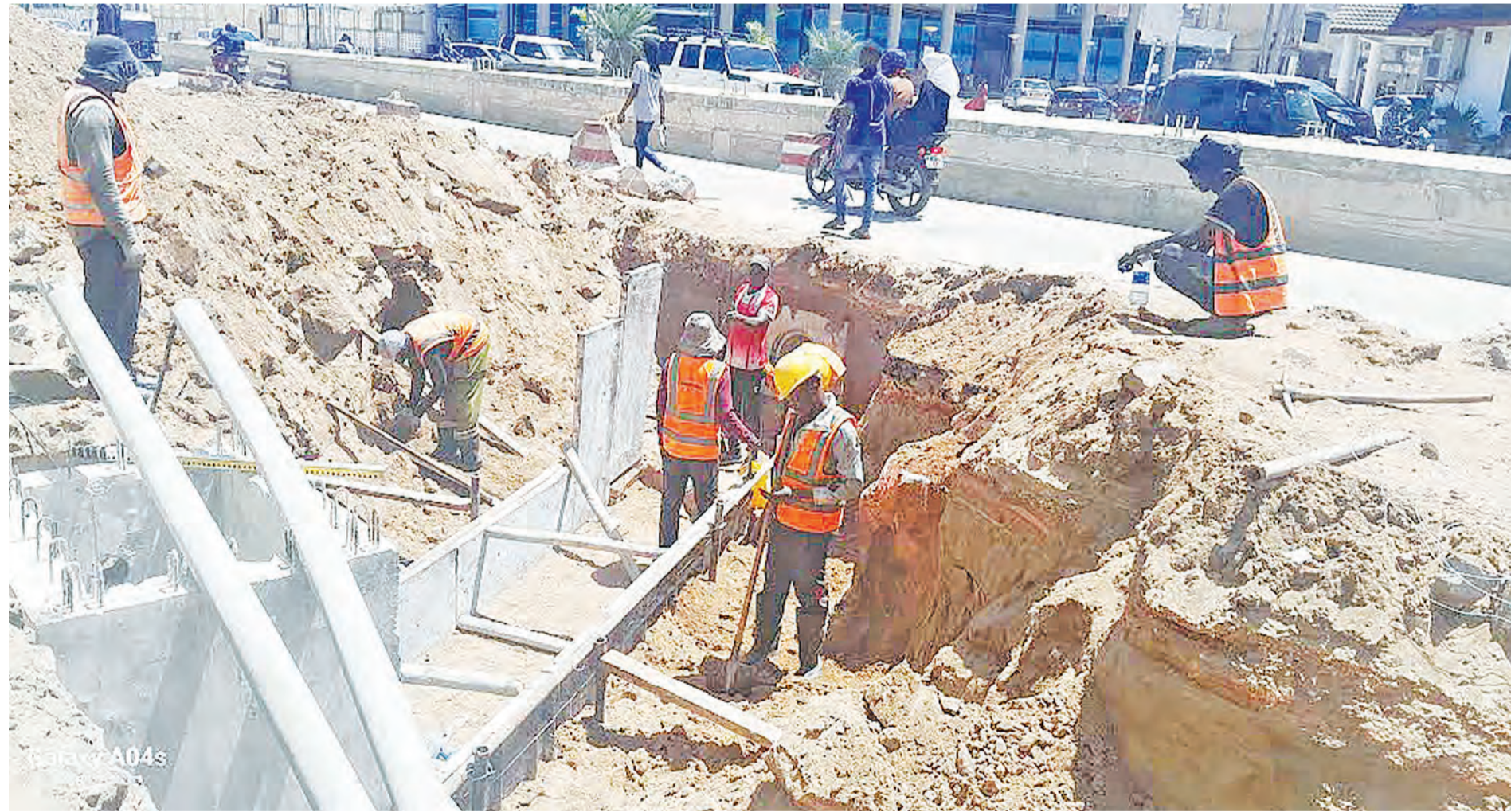
Contractor workers in progress of the rain water drainage system construction along Bibi Titi Mohamed Road in Dar es Salaam yesterday. Photo: Correspondent Imani Nathaniel.
