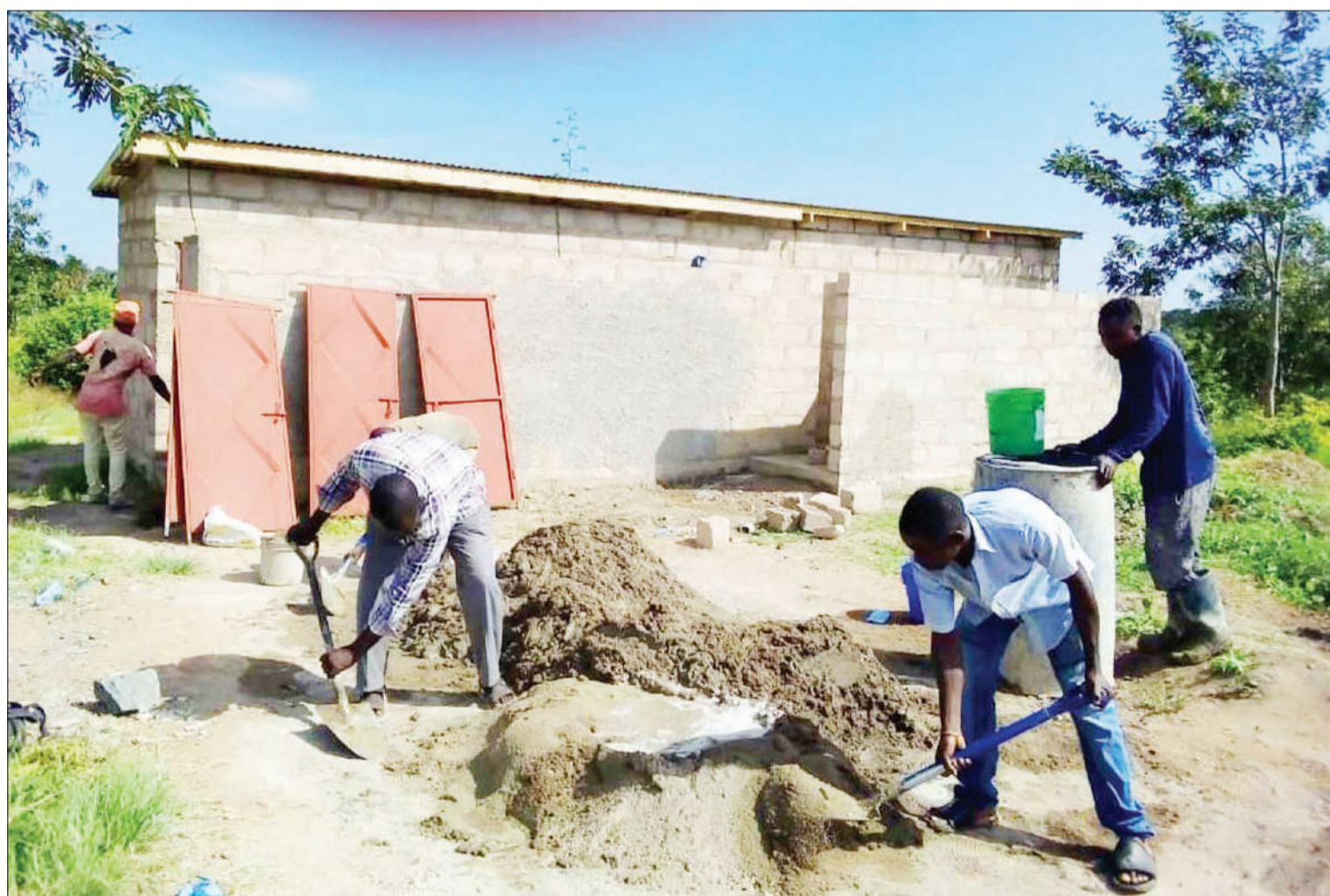
Work on a new toilet building in progress at the weekend at Kigera Secondary School in Musoma Rural constituency. The school is expected to enrol its first Form One class later this month. Photo: Guardian Correspondent
