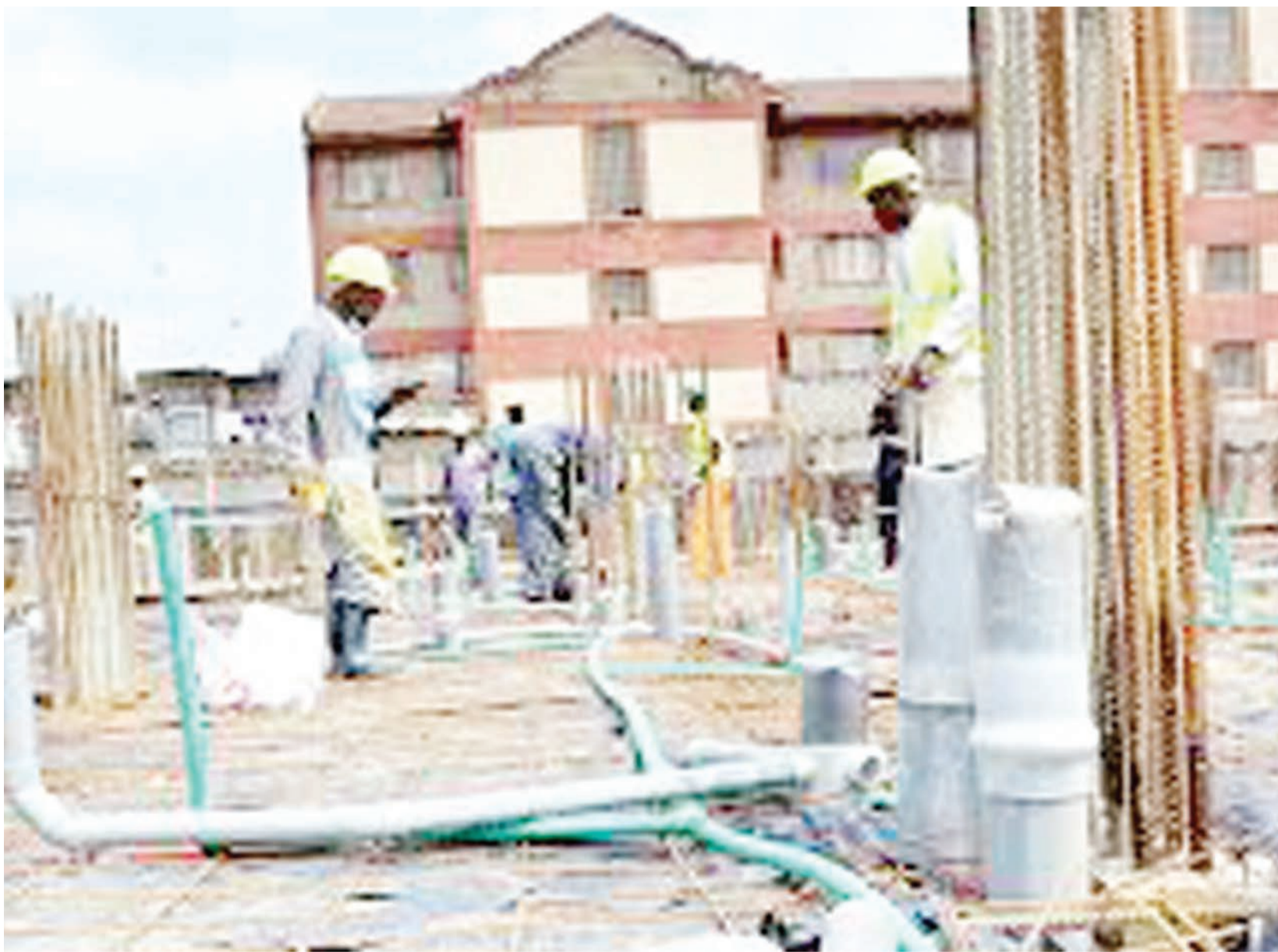
Workers at a housing construction site in Nairobi. The Kenyan Government aims to deliver 500,000 units in major towns across the country over the next four years.
