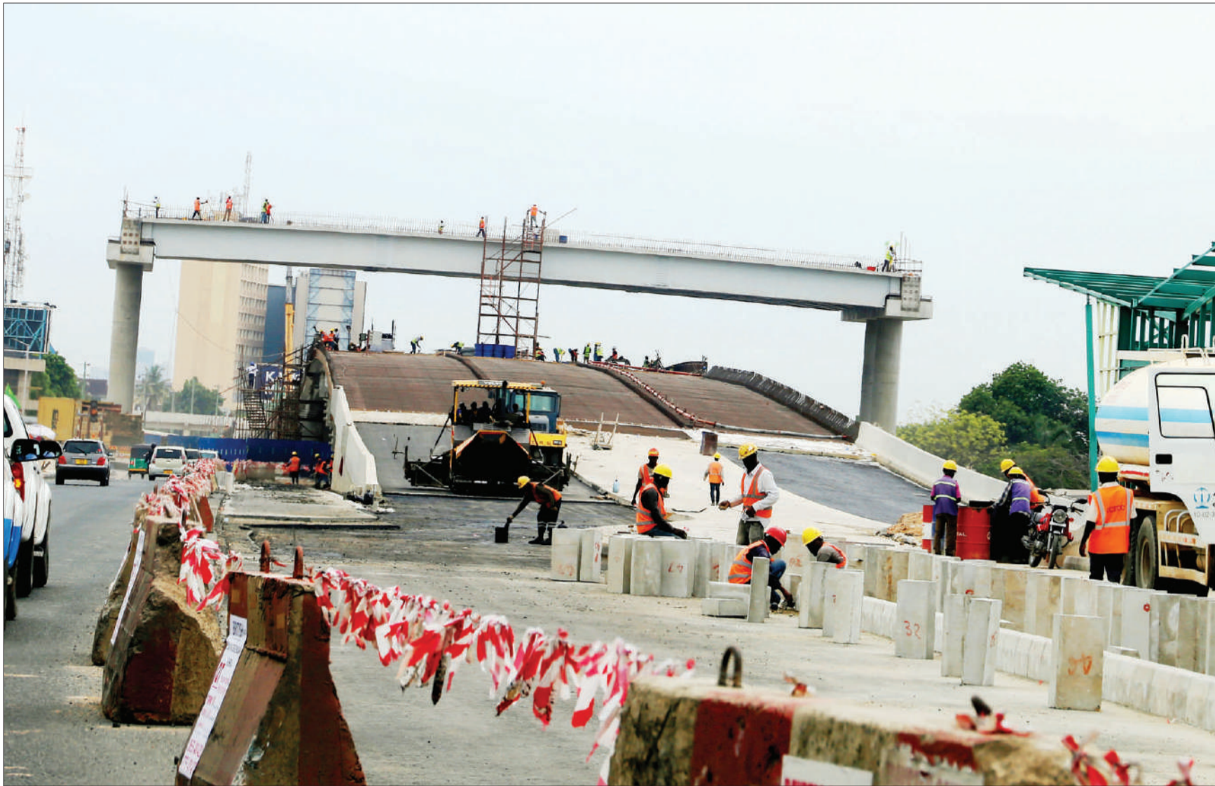
Ubungo interchange flyover project is going on well as the Chinese company employees work on three lanes as captured yesterday. Photo: Guardian Photographer
