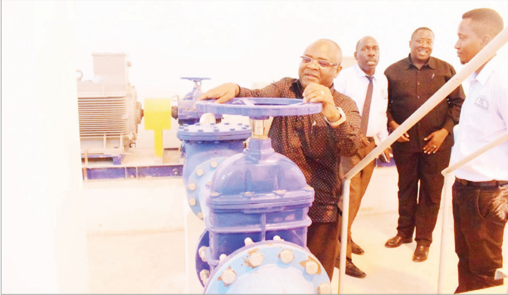
Permanent Secretary in the ministry of Water Prof. Kitila Mkumbo (2nd R) inaugurates Salasala water project implemented by the Dar es Salaam Water and Sanitation Authority (DAWASA) in Dar es Salaam yesterday. Looking on is Dawasa Chief Executive Officer Cyprian Luhemeja (2nd R) Photo: Guardian Correspondent
